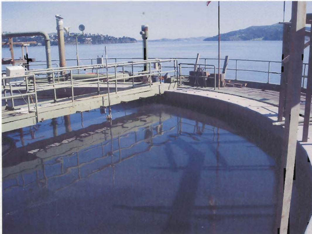
Figure 3: Primary clarifier. Note covered weir.
