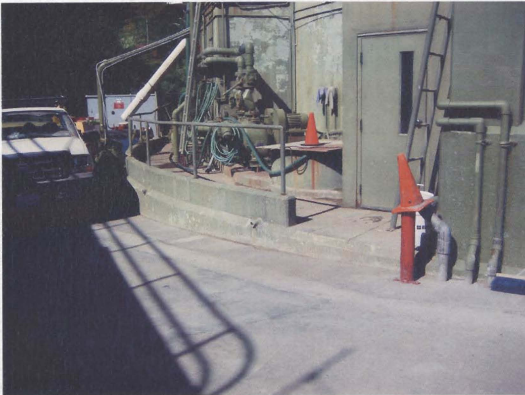
Figure 13: Digester located beneath primary clarifier.
