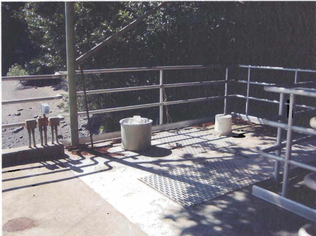
Figure 8: "Water Champ" chlorination point.
