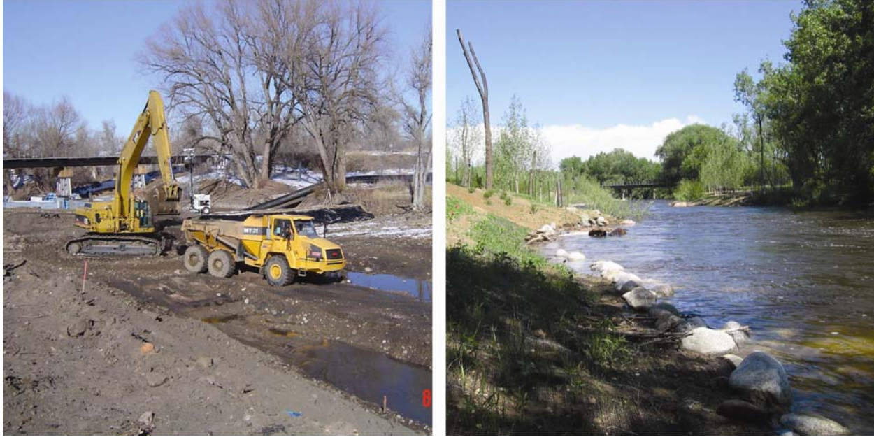
Figure 5-1: Before and after photographs of the Cache La Poudre River Superfund Site in Colorado, where EPA implemented an ecological remedy to preserve the riverine habitat and restore the streambank. See Appendix A for additional information. Photographs courtesy of Paul Peronard, EPA Region 8.
