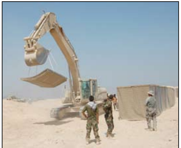
Afghan National Army soldiers assigned to 4th Kandak, 3rd Brigade, place barriers during construction of a new expeditionary forward operating base.
