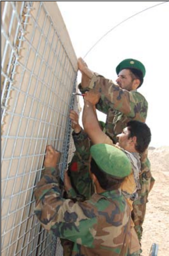
Afghan National Army soldiers, assigned to Afghan National Army’s 4th Kandak, 3rd Brigade, mesh portions of a barrier together during construction of a new expeditionary forward operating base. The base will be built and maintained by the ANA.
