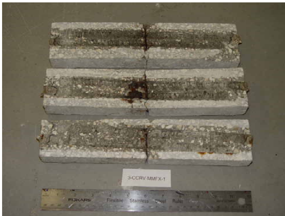
Figure 4.65. Photo. Trace of the upper rebars and corrosion products on specimen number 3-CCRv-MMFX-1.
