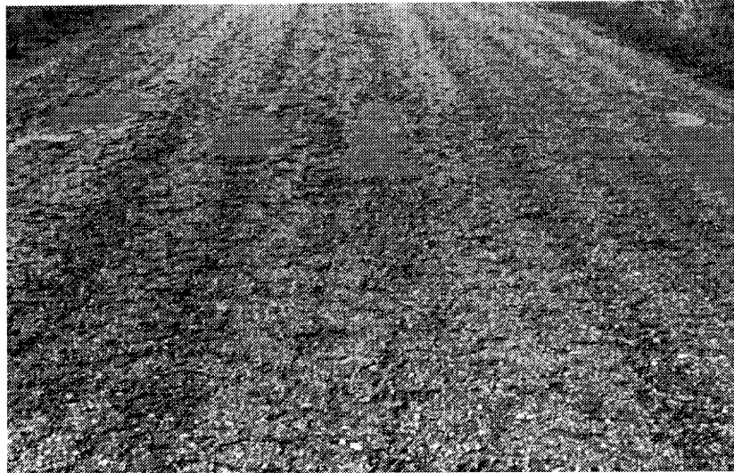
Figure 2-1. Example of severe surface ravelling. (1)
