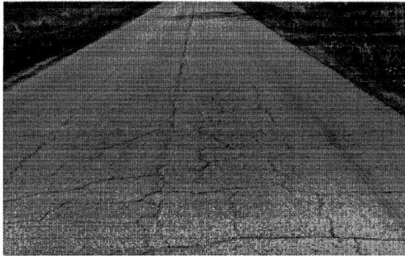
Figure 2-4. Example of intermediate-sized block cracking. (1)
