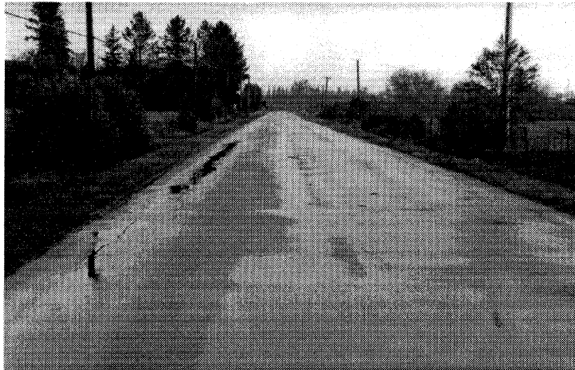
Figure 2-5. Example of slight to moderate rutting. (1)
