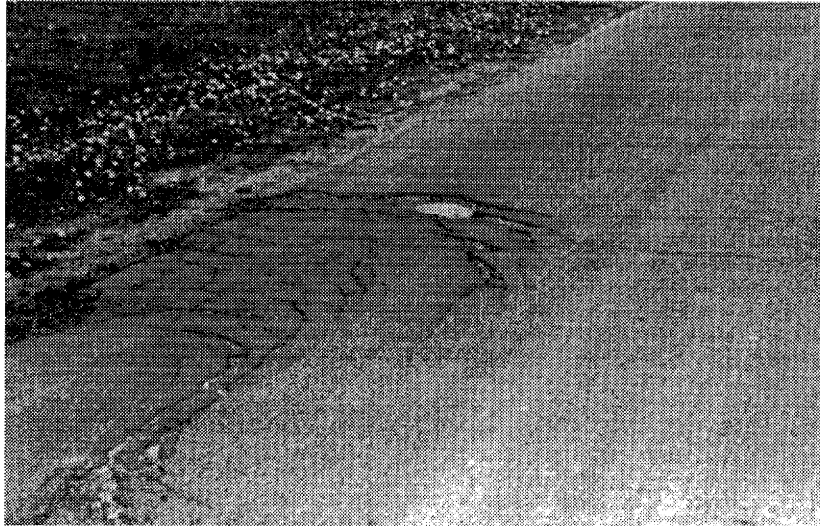
Figure 2-3. Example of slippage cracking. (1)
