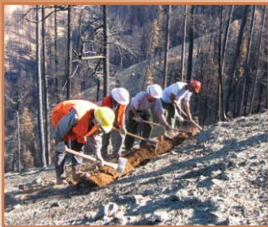
Researchers are comparing the effectiveness of postfire treatments for reducing erosion and regenerating vegetation. The first step is digging a trench on a slope's contour after a wildfire and then installing a silt fence to capture sediment (Umatilla National Forest).
