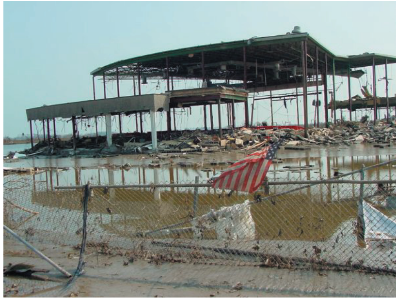
Figure 12. Damage from Hurricane Rita in Cameron, LA
