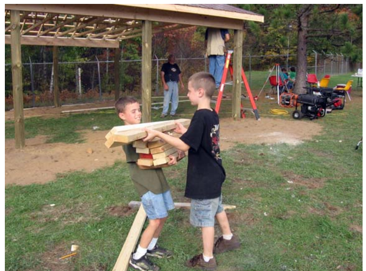
-USFWS Even the "Kids of the Friends" pitched in to help get the Visitor Pavilion constructed at the hatchery.
