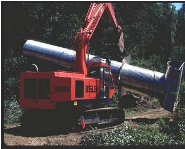
Road Maintenance. Culvert installation under road bed to prevent flood damage. USFWS.
