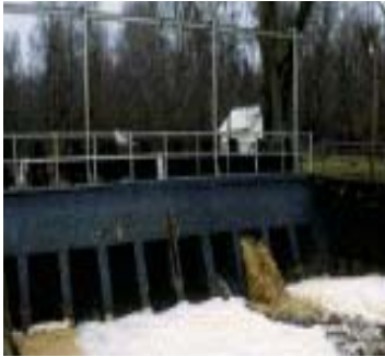
Lake Drummond Spillway. Water control spillway releasing into the Feeder Ditch. USFWS.
