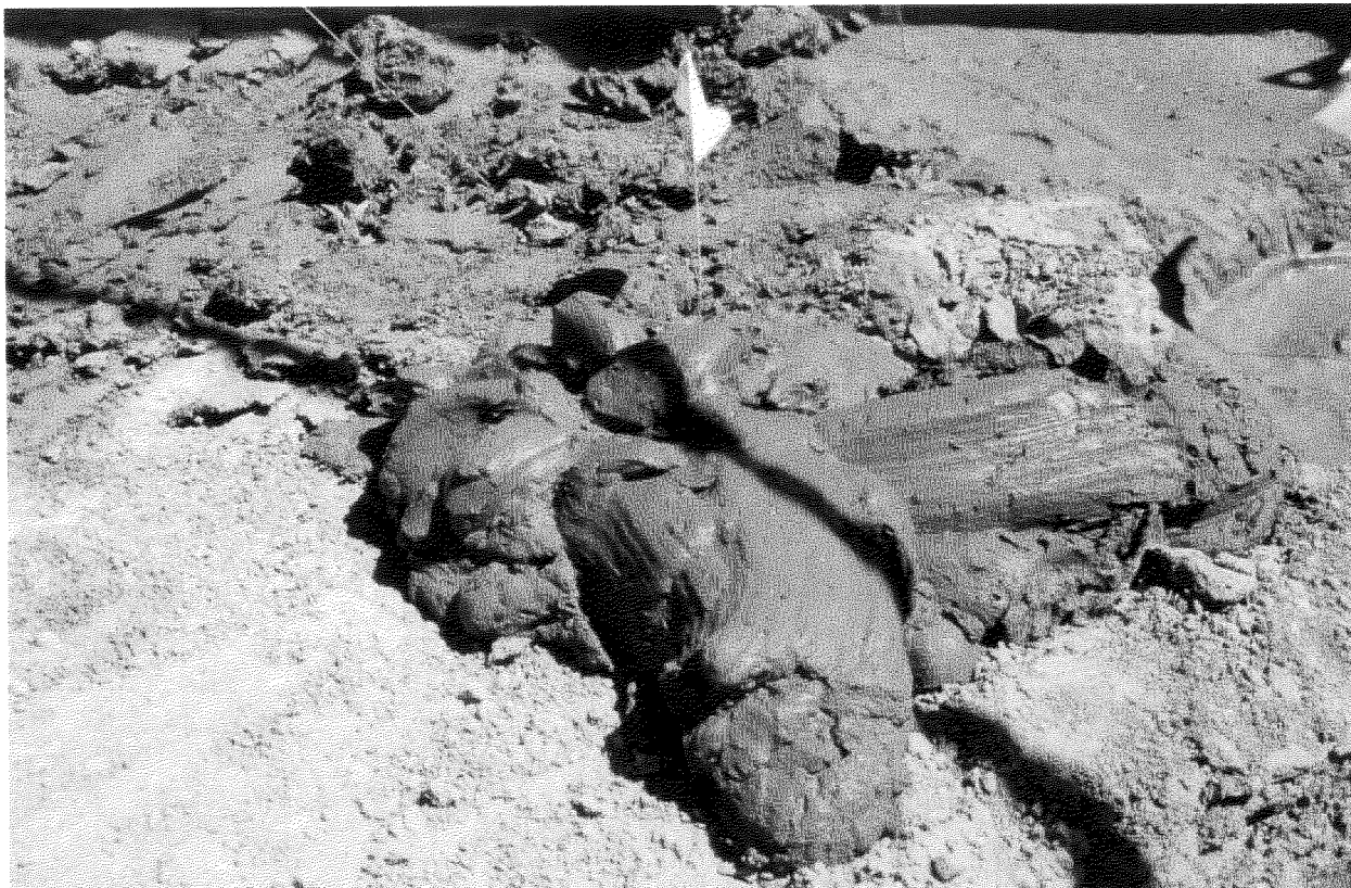
Figure B-3. Excessive grout returns caused by low soil porosity.
