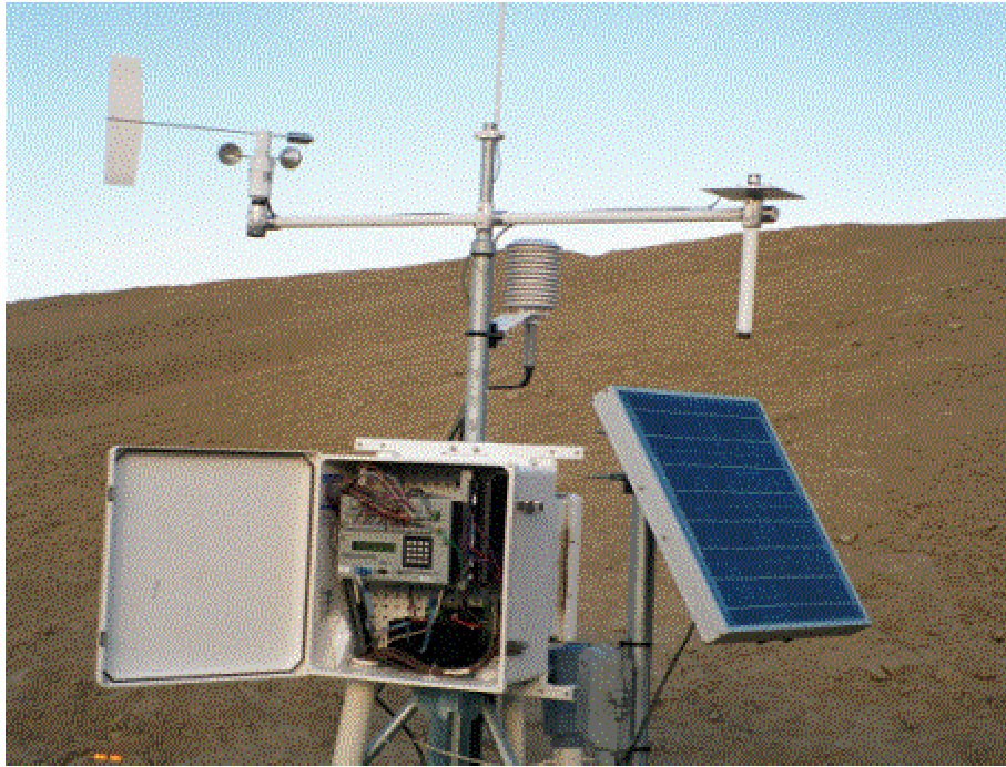
Figure 4. Typical instrument installation.ACAP
