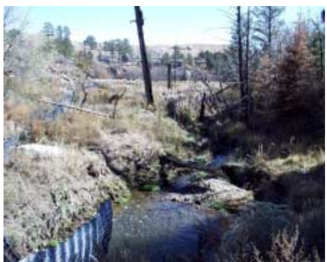
Figure 5b: A 2000 photograph of upper Sandia wetland at the culvert showing an incised stream channel and increased sedimentation below the sediment fence.
