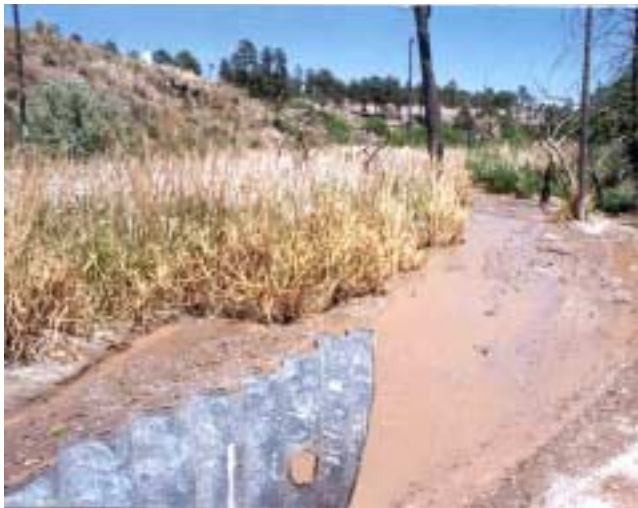
Figure 5a: A 1990 photograph of upper Sandia wetland at the culvert by the rubble landfill showing a wide, diffused (braided) stream channel with cattails.
