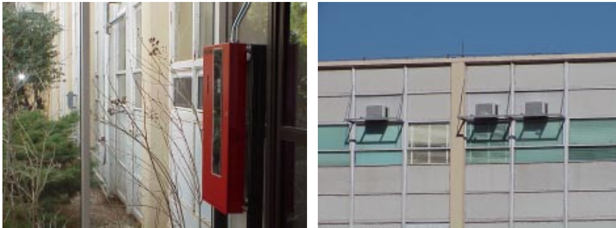
Figure 3c. Exterior fire alarm panel and air conditioning units.
