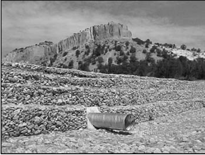
The low-head weir across Los Alamos Canyon will contain contaminated sediment. (Photo courtesy of Sacramento District)
