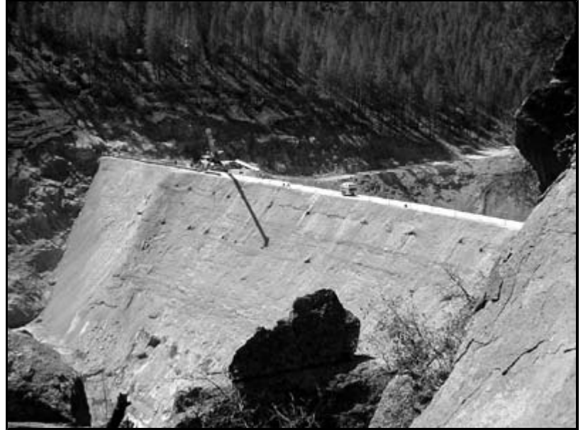
The flood retention structure at Pajarito Canyon will protect Los Alamos Technical Laboratory. (Photo courtesy of Sacramento District)
