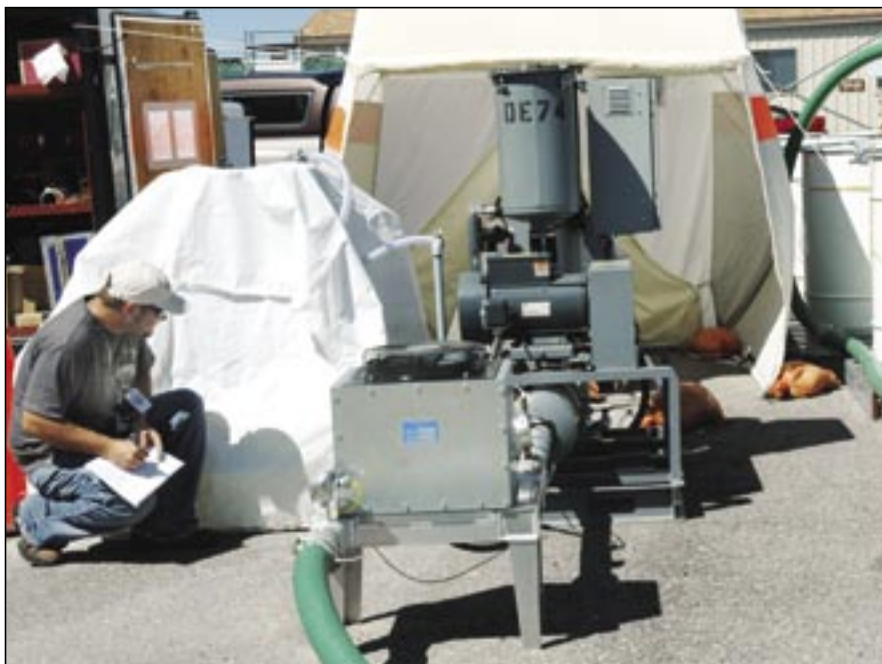
William Stewart, an environmental engineer with Apogen Technologies, gathers data from the soil-vapor-extraction apparatus that is cleaning up a subsurface solvent-vapor plume at Material Disposal Area L, a former disposal area at TA-54. Photo by James E. Rickman
