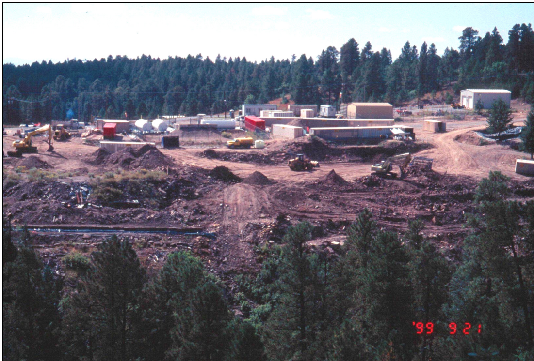
Photograph 2.2-2. Excavation activities in the west lob of MDA P, 1999 (view to south)
