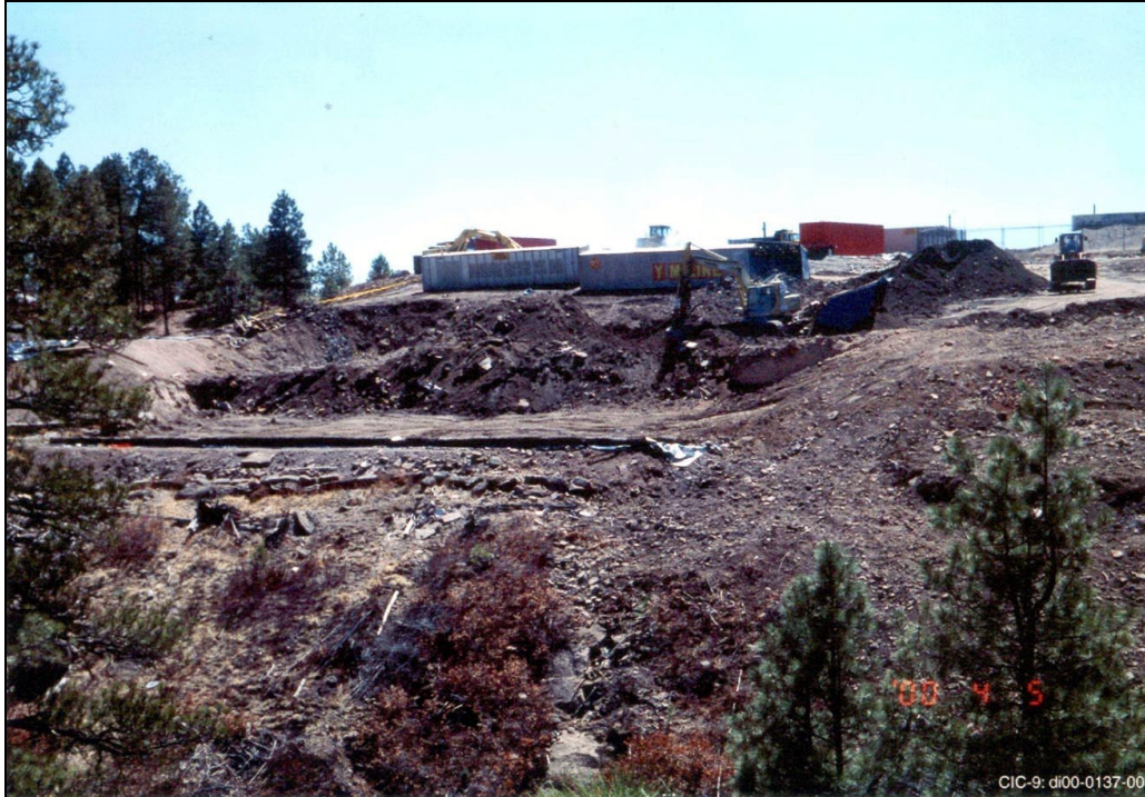
Photograph 2.2-3. Excavation activities in the east lobe of MDA P, 2000 (view to south)
