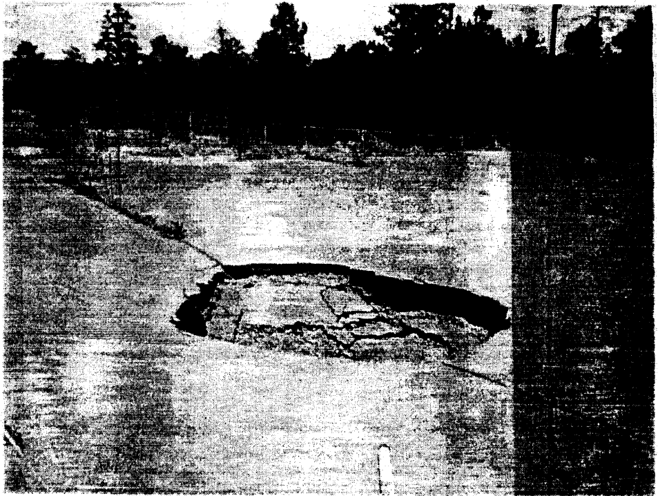
Figure 7.3-2 Appearance of the collapsed section of asphalt over Area 2 in 1975, viewed to the west. Hole area was about 3 ft by 6 ft and the depth was about 3 to 4 ft.
