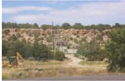
White Rock Substation
