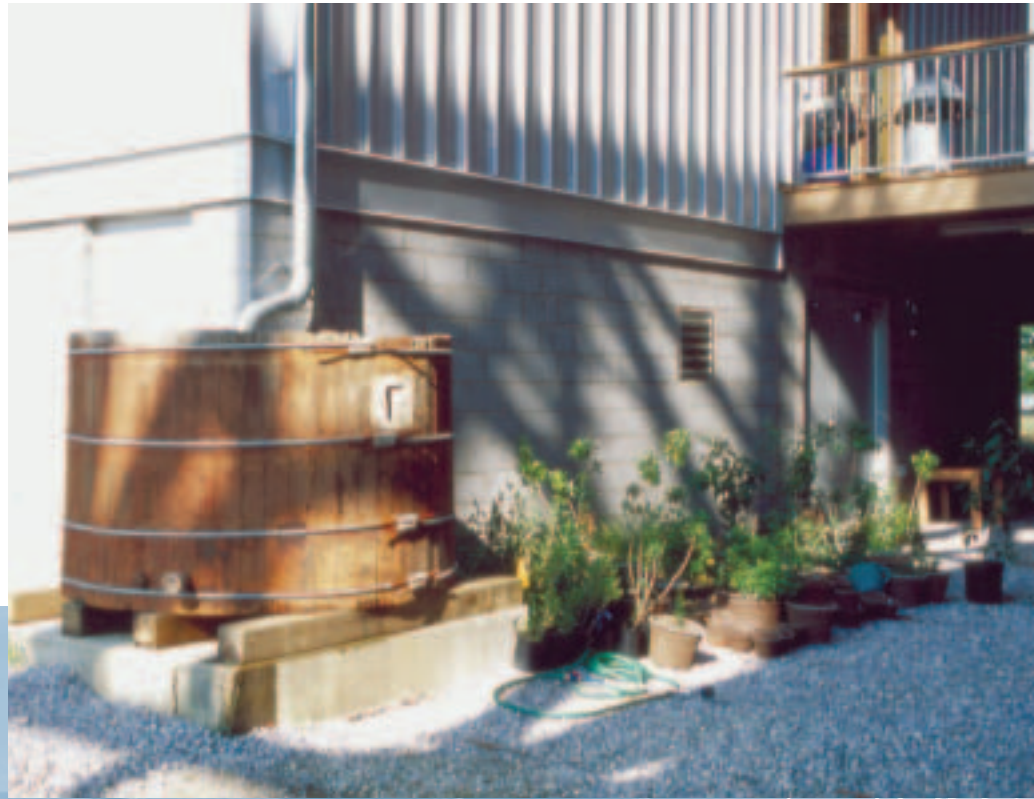
A small cistern stores rainwater for landscape irrigation at the Chesapeake Bay Foundation's Phillip Merrill Environmental Center in Annapolis, Maryland.
