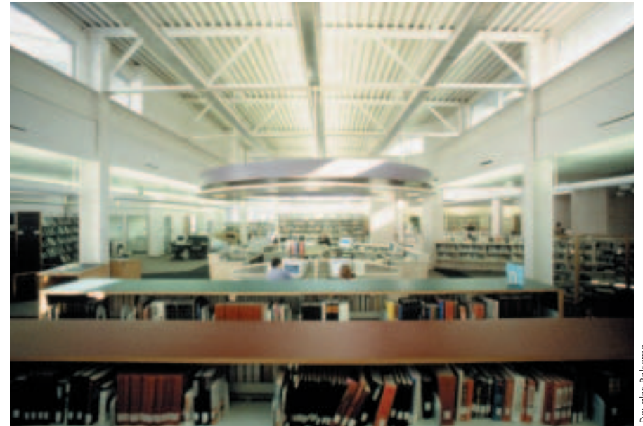
Photo sensors control the dimmable electric lighting to supplement the available daylight and maintain constant illuminance levels within the Harmony Library in Fort Collins, Colorado.
