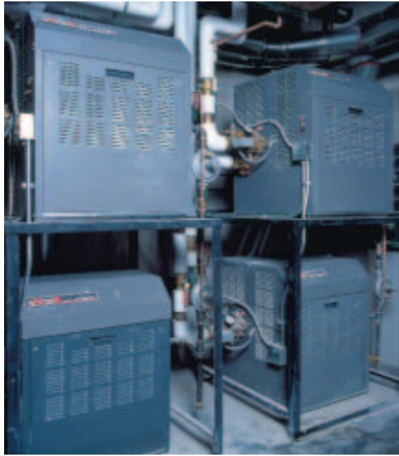
Modular boiler system provides good part-load efficiency and redundancy.
