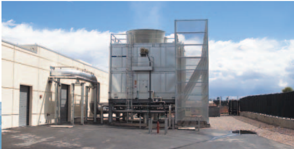
The LANL Nicholas C. Metropolis Modeling and Simulation Center currently uses treated wastewater from the LANL complex for cooling tower application.
