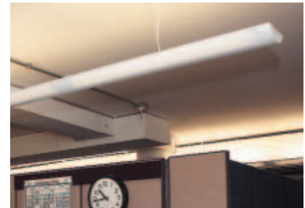
Indirect lighting fixtures with T-5 lamps in the LANL PM Division offices reduces glare and provides more uniform ambient light.
