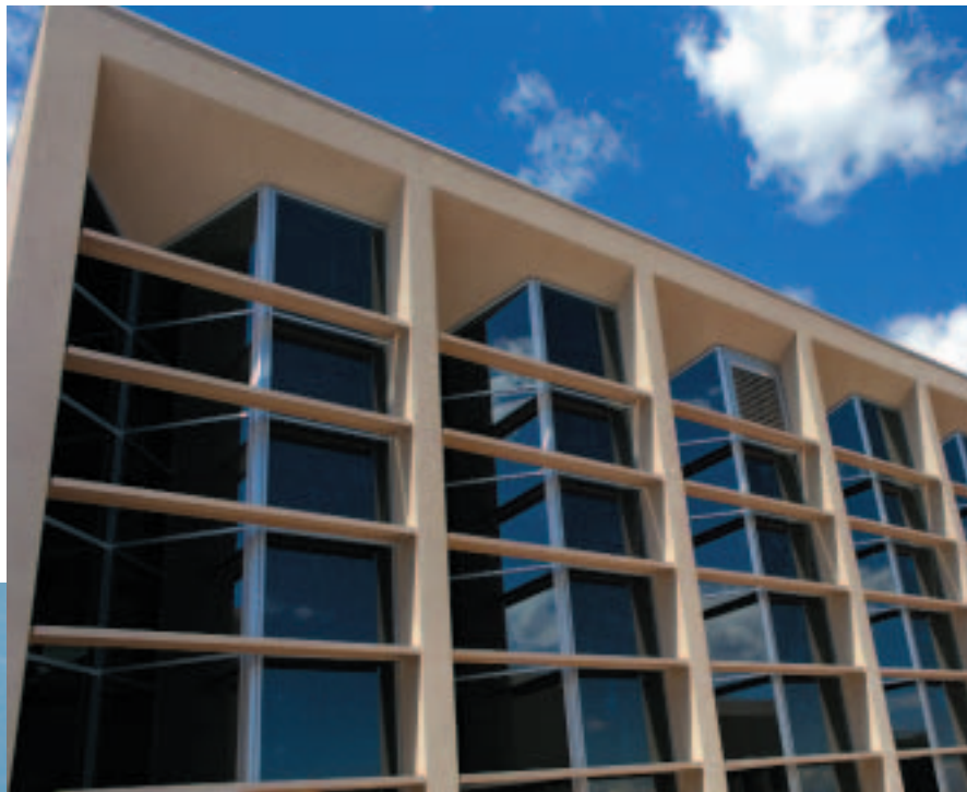
This Trombe wall design incorporates windows to provide daylighting. Horizontal elements in front of the Trombe wall shade it during summer.
