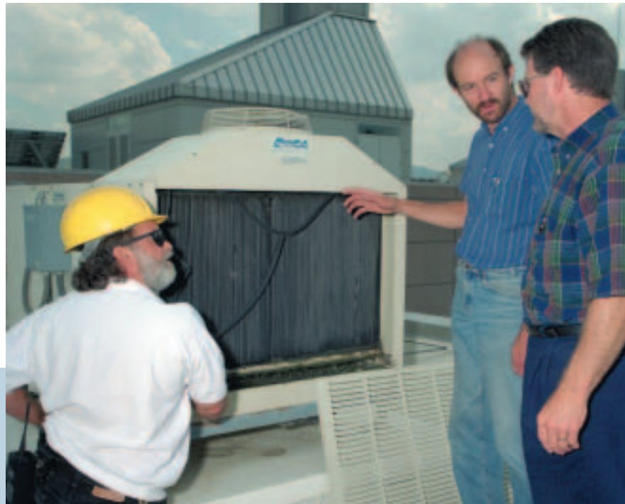
Rooftop cooling equipment inspection with building owner representative, facility engineer, and installer.
