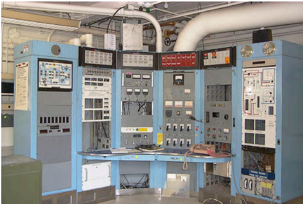
Figure 14.5. Omega West Reactor Control Panel at TA-2.
