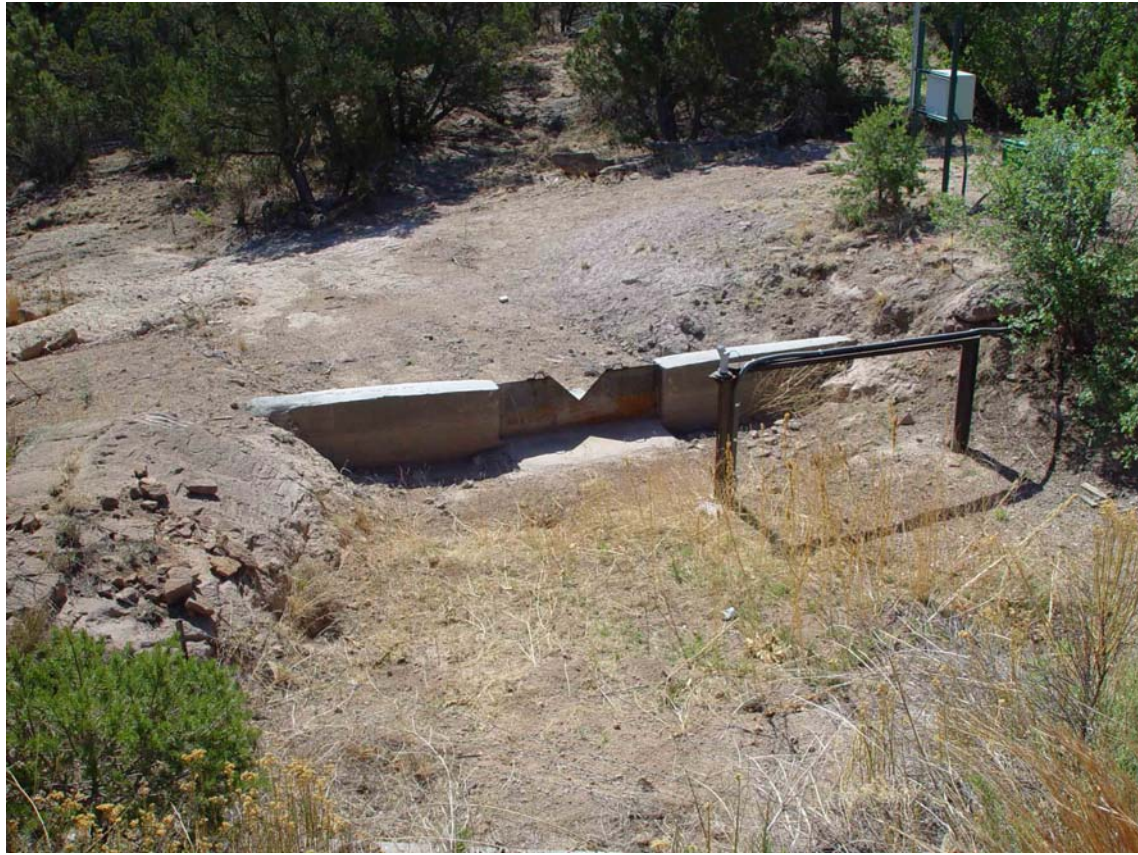
Photo 70-5: The head of the ravine where it crosses SR4 has a metering station that can provide flow data.
