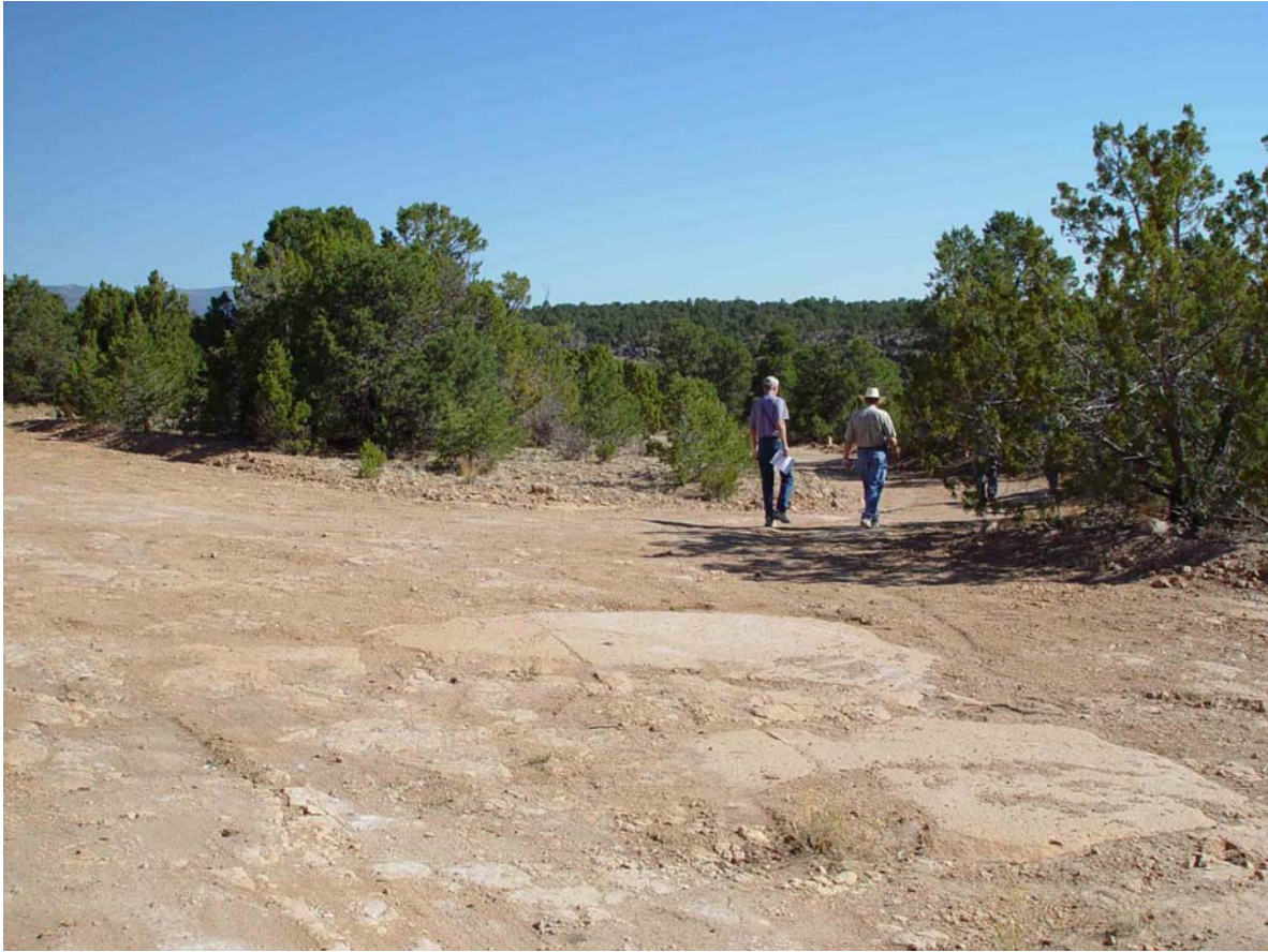
Photo 49A-1: The road on top of the mesa before entering the ravine is built on tuff and is relatively flat.
