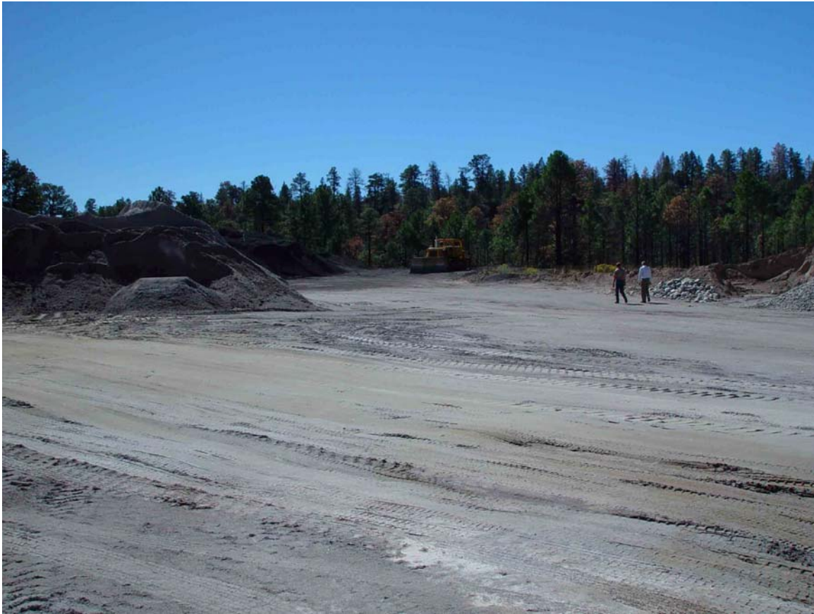
Photo 61-3: A view to the south. The tractor in the background lies close to the edge of the canyon, and shows the approximate southern limit of the landfill site. The trees on the horizon are located on Sigma Mesa (TA-60), across Sandia Canyon.
