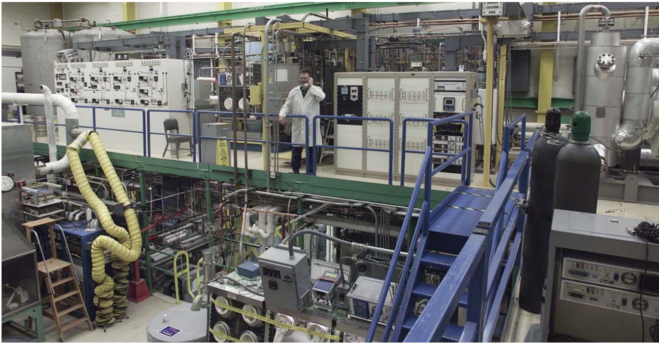
Power Plant Complex
