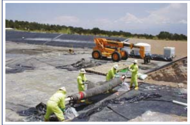
Removal of dried radioactive sludge and the plastic liner from a lagoon at LANSCE.
