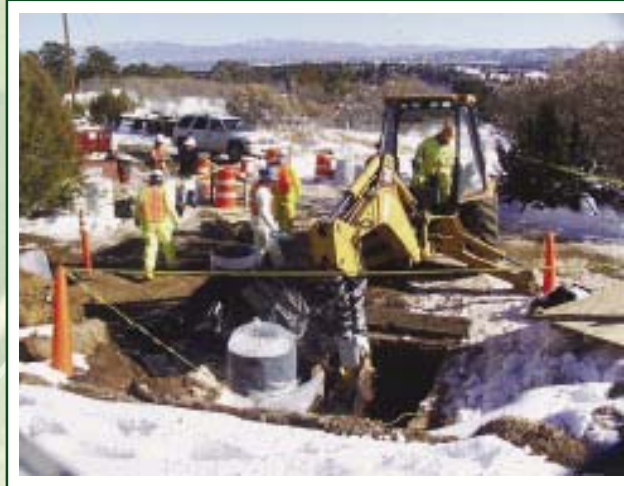
Septic tank removal activities at Technical Area 21 on the edge of Los Alamos Canyon.
