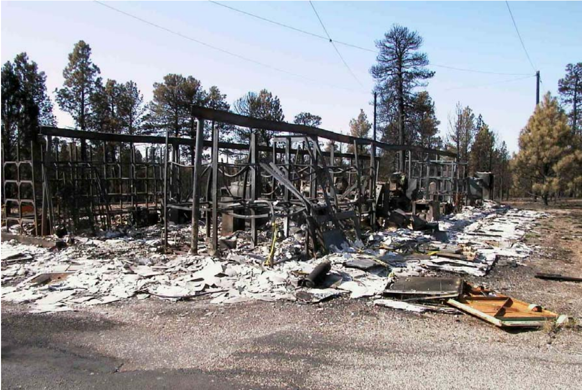
Figure 11.14. TA-40-73 after the Cerro Grande Fire.
