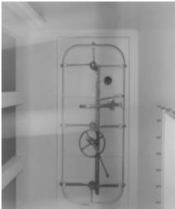
Figure 4.37 – Filter Plenum (Door-Wheel Style)
