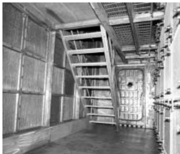
Figure 4.6 – Man-entry Two-Level Plenum (lower level) (Looking at Mist Eliminator Upstream Side of First HEPA Filter Stage)
