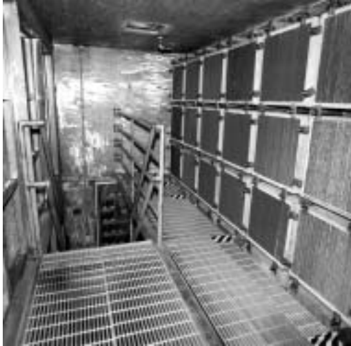
Figure 4.7 – Man-entry Two-Level Plenum (Upper Level Looking at Upstream Side of First HEPA Filter Stage)
