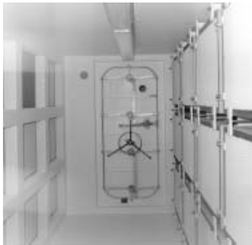
Figure 4.8 – Man-entry Plenum (Looking at a Ship Door Between HEPA Filter Stages)
