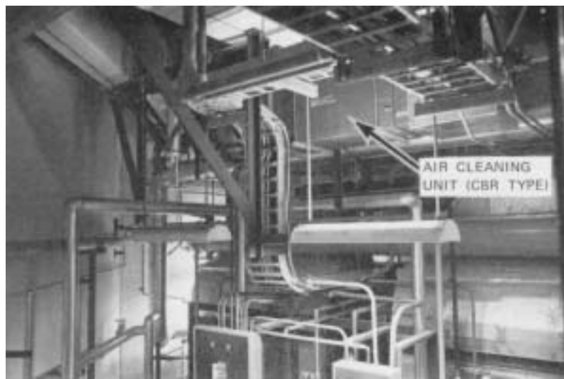
Figure 2.13 – An Illustration of Poor Filter Installation Practice
