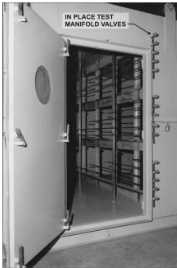
Figure 4.33 – Filter Plenum Entry Door (No Airlock Type-Test Manifold with Valves Shown)
