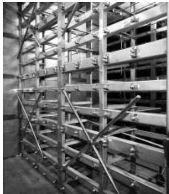
Figure 4.12 – Adsorber Tray Mounting Frame (“X” Cross Units Are for Test Gas Injection)
