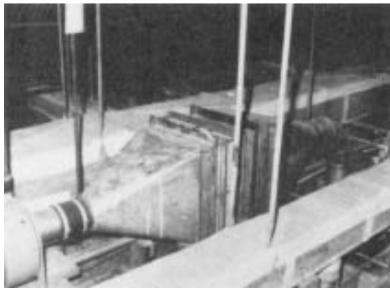
Figure 2.12 – An Illustration of Poor Filter Installation Practice
