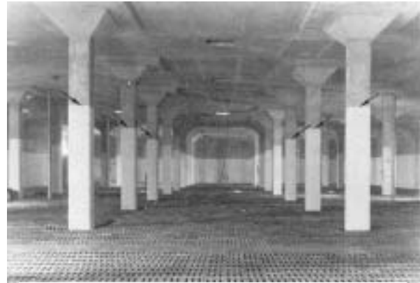
Figure 9.4 – Interior of New Sand Filter at Savannah River Laboratory Before Loading of Sand and Aggregate
