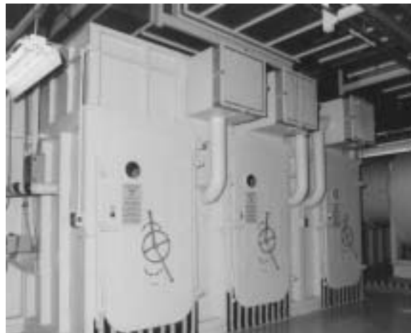
Figure 4.5 – Airlock Entry for Man-entry Plenum (Filters Above Doors are to Allow Pressure Equalization)
