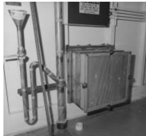
Figure 4.40 – Filter Plenum Drain P-Trap Fill Tube
