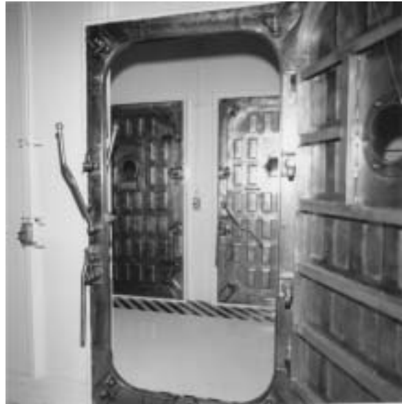
Figure 4.36 – Filter Plenum (Looking from Outside into the Airlock at the Final Stage Upstream and Downstream Doors)
