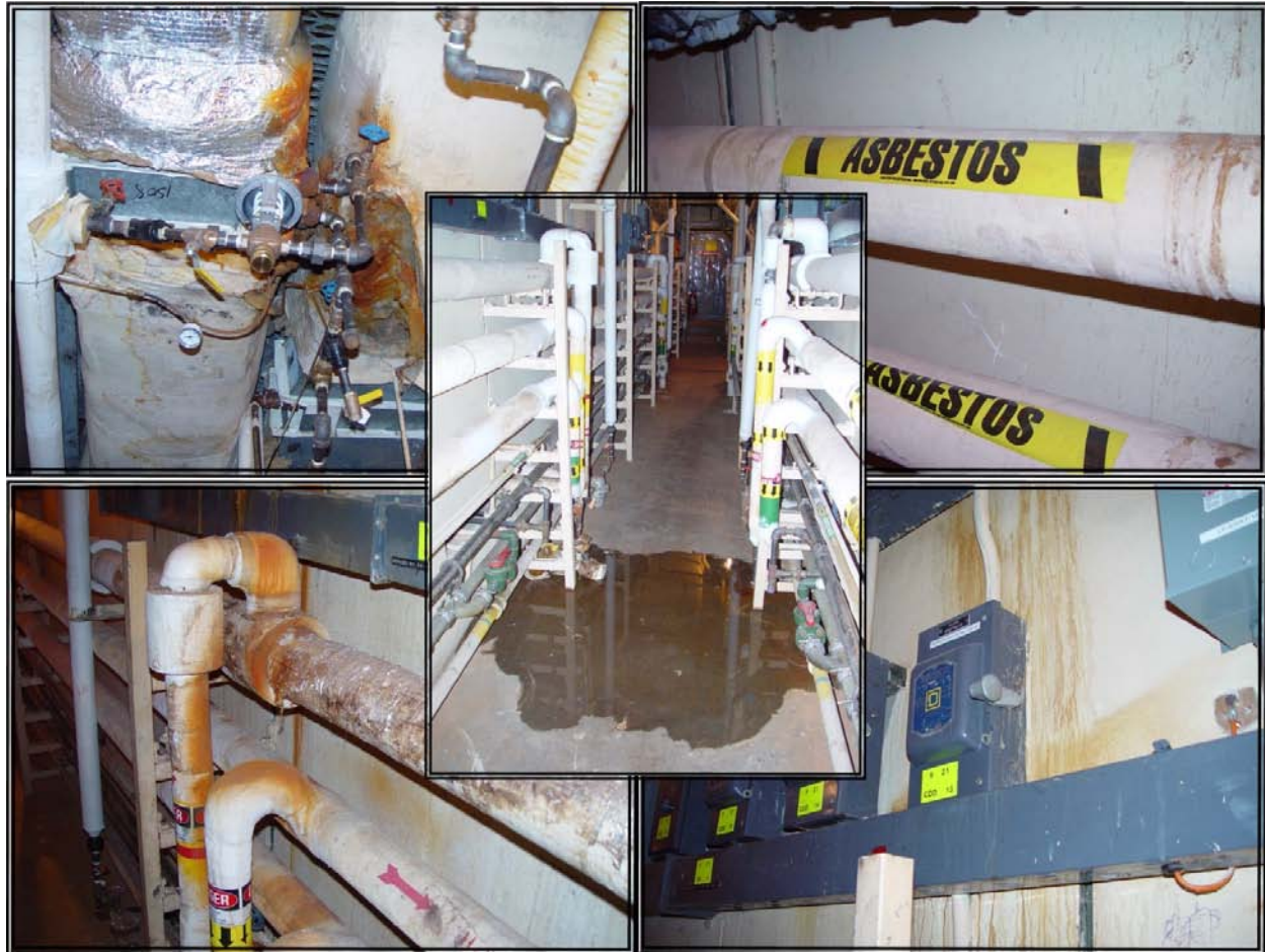
Photo 2. Maintenance problems at DX facilities.
