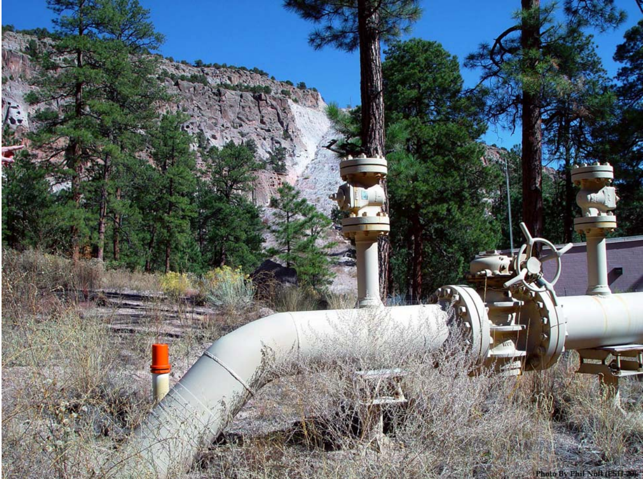
Figure 3. Existing aboveground 12-in. (30-cm) PNM gas mainline valve in Los Alamos Canyon.
