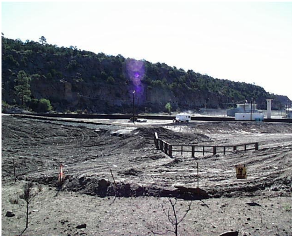
PHOTO 2.22—Trash Rack above TA-18 with Steel Diversion Wall in Background
