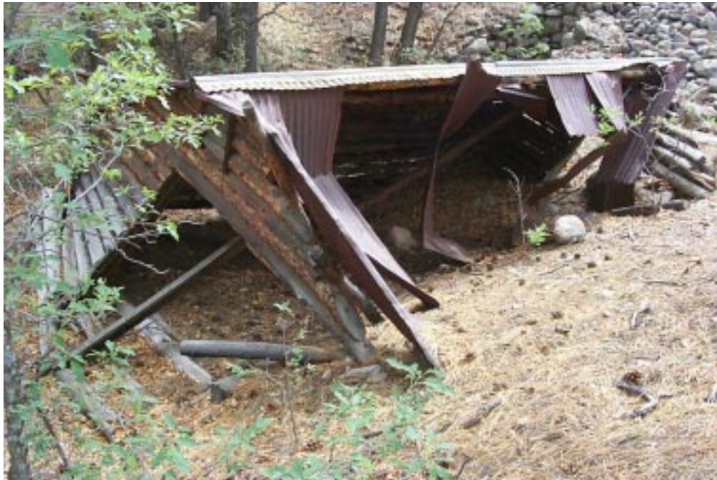
PHOTO 3.5—Anchor Ranch Icehouse before June 28, 2000, Flooding
