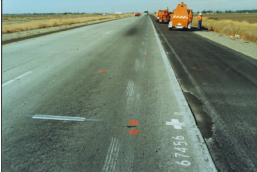
Figure 4.3.1 Overview of the experimental test road at Tracy. Thickened test section 06-7456 with low distress levels.
