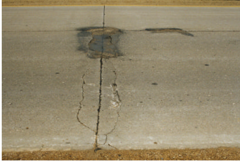
Figure 4.4.2 Spalling crack running parallel with the joint in a distance of about 0.3 m.
