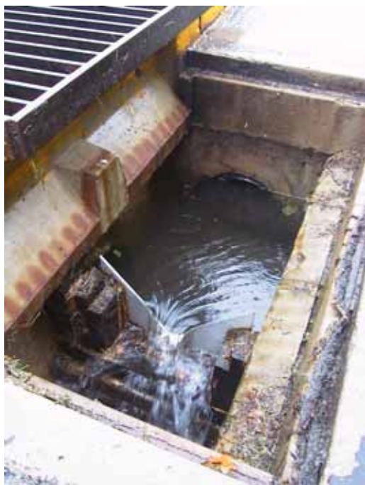
FIGURE 5-54 Weir flow used to measure flow rate. Courtesy of Robert Traver.
