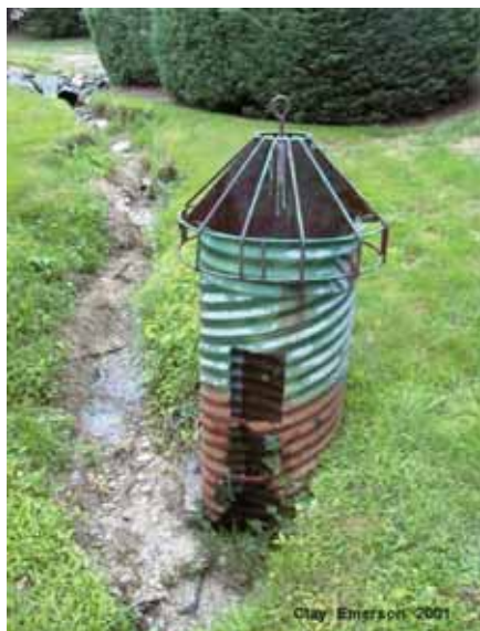
FIGURE 5-50 Rusted outlet structure. SOURCE: Reprinted, with permission, from Emerson. Copyright by Clay Emerson.
