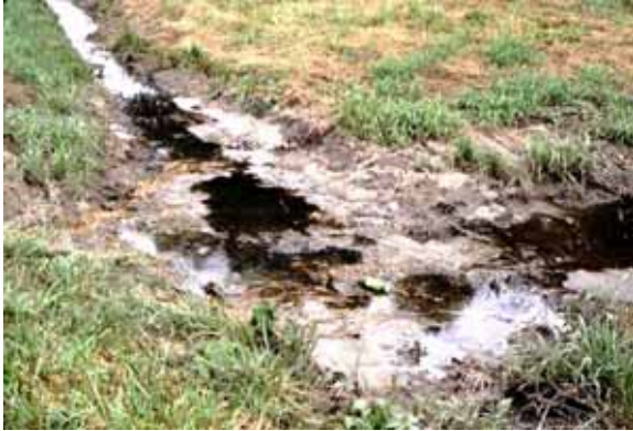
Failing sanitary sewer, causing upwelling of sewage through soil, and draining to gutter and then to storm drainage system.
