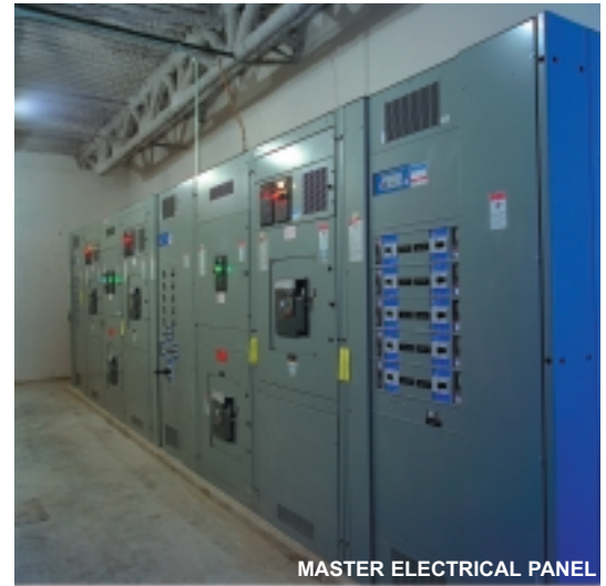
MASTER ELECTRICAL PANEL
