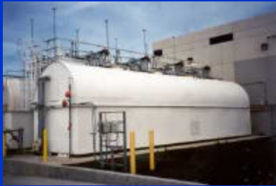
Sheltered above ground tank farm
