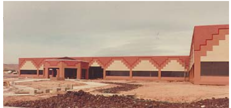
Above: The IHS Hospital in Chinle, AZ, under construction, showing the hogan design entrance. Right: The interior courtyard and waiting area of the Chinle IHS Hospital. Special stone work creates an environment that is appealing to the patients and family members who use this facility.
