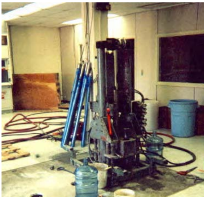
Figure 4-5. Indoor Direct Vibra-Push™ Rig (LD Geoprobe® Series) Used in the Engineering Support Building
