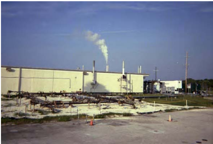
Figure 3-2. Steam Injection System in Operation at Launch Complex 34
