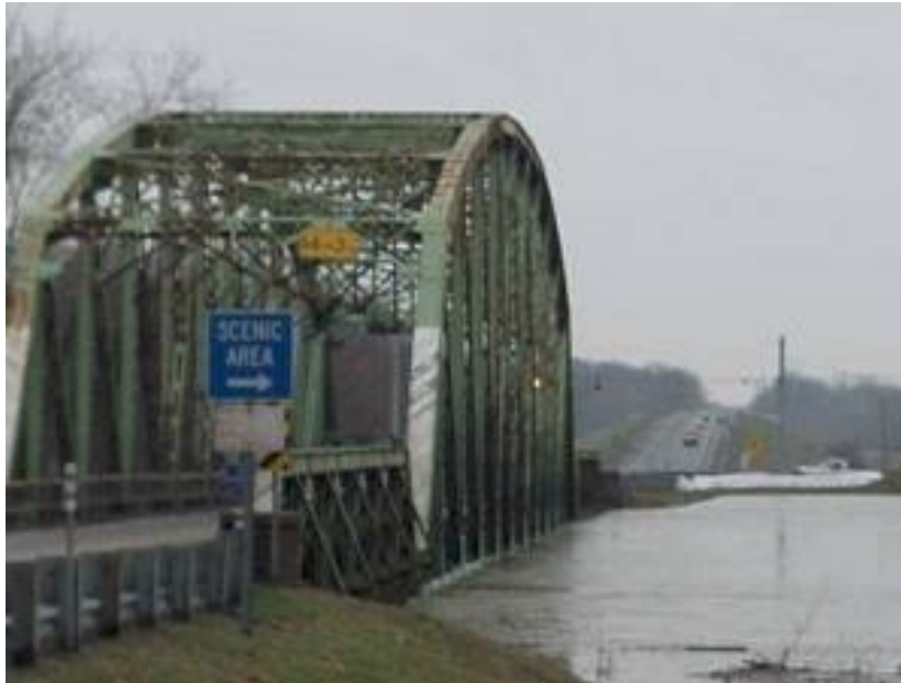
Photo of the State Route 64 bridge over the Wabash River at East Mount Carmel, IN on January 11. Photo supplied by Amy Lindsey, Indiana State Emergency Management Agency.
