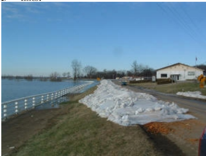
Photo of the makeshift levee constructed on U.S. Highway 60 in Smithland, KY. The highway was closed to eastbound traffic for over a week. With no permanent levee, a makeshift levee is built to protect Smithland during each major river flood. Photo taken on Route 60 at the Smithland city limits. Photo courtesy of Jeff and Christine Wielgos.
