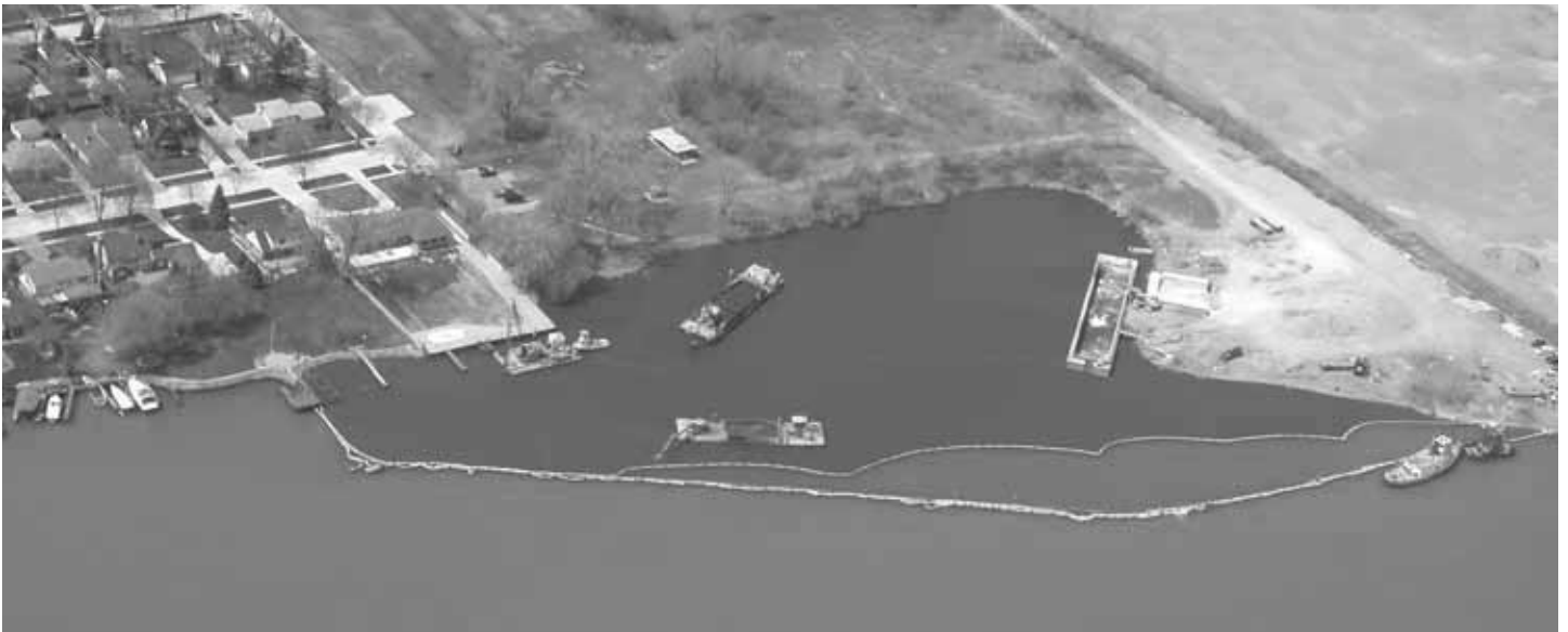
This photo shows the silt curtain that was constructed around the Black Lagoon to keep resuspended sediment from entering the river.
