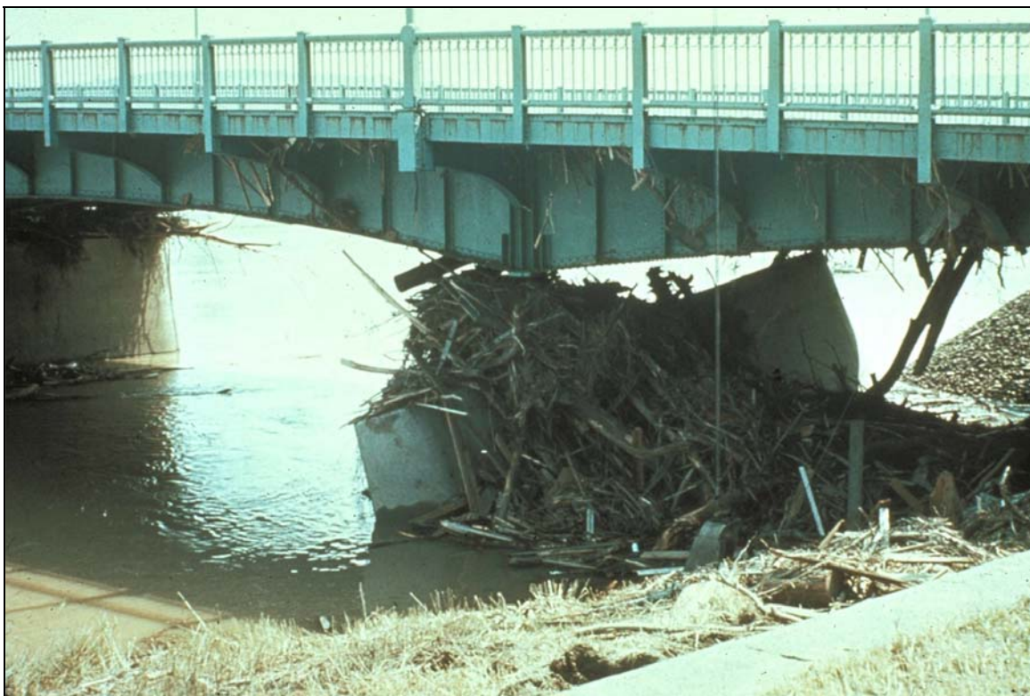
Figure 2.2. Single pier debris accumulation (led to pier scour failure).
