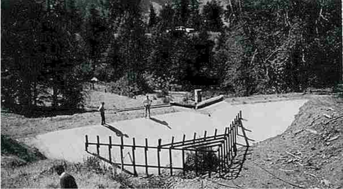
Figure 5.40. Debris dam and basin along with steel debris rack over culvert entrance in foreground. A metal pipe riser is visible over the spillway.
