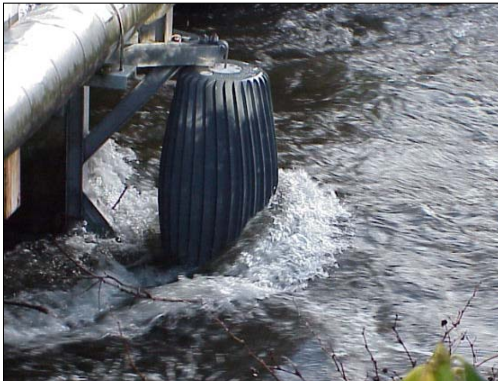
Figure 5.45. Close up of a debris sweeper installed on the Cedar Creek in Washington.
