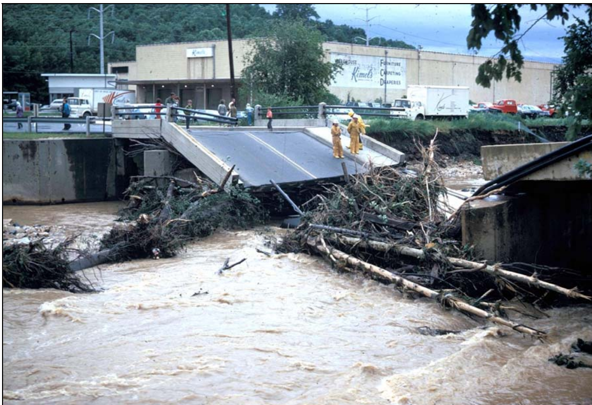
Figure 2.8. Effects of debris accumulation at a bridge structure. (New York)
