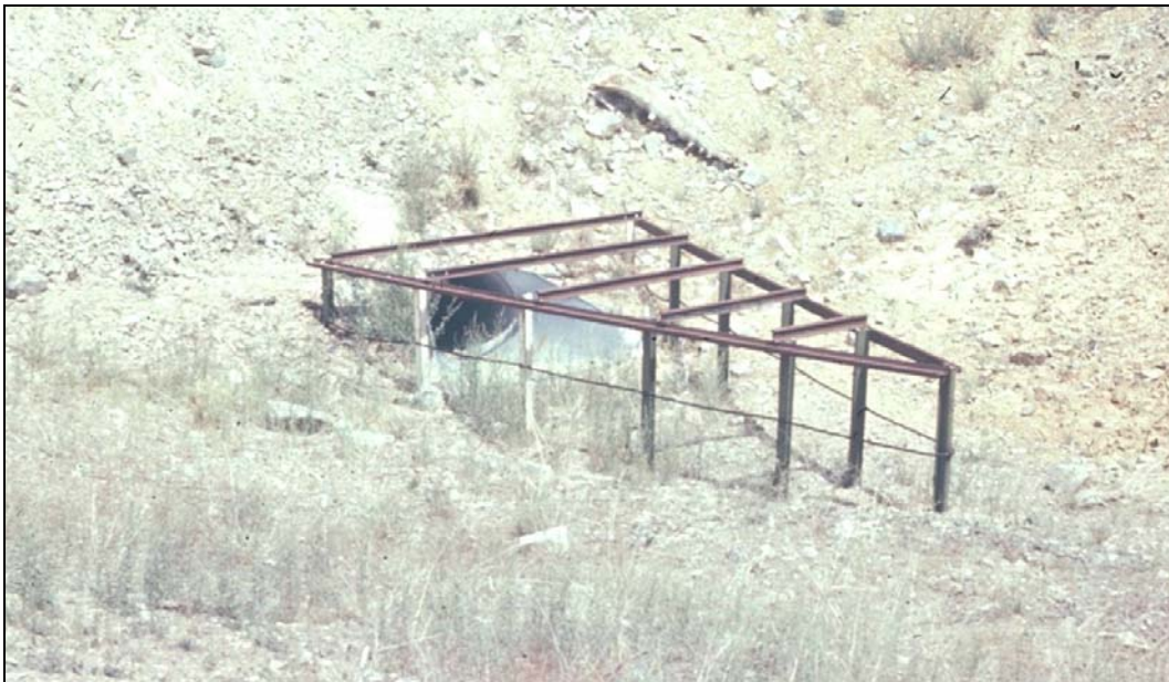
Figure 5.3. Steel rail and cable debris deflector. In boulder areas, cable is more desirable for its flexibility than a rigid rail (looking towards entrance).
