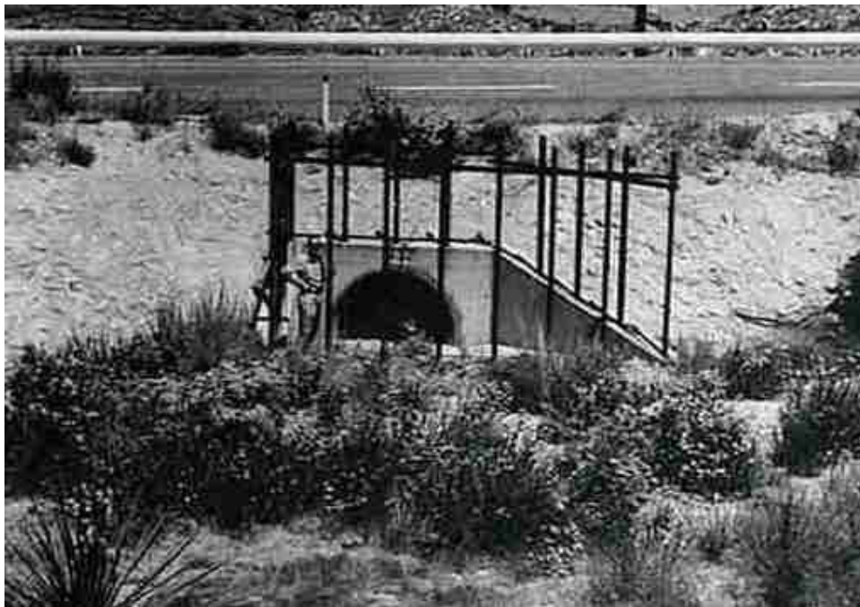
Figure 5.18. Installation in Figure 5.17 after several years of fine silt deposition at entrance.
