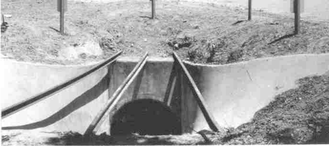
Figure 5.10. Rail debris rack over sloping inlet. Heavy debris and boulders ride over rack and leave flow to culvert unimpeded.
