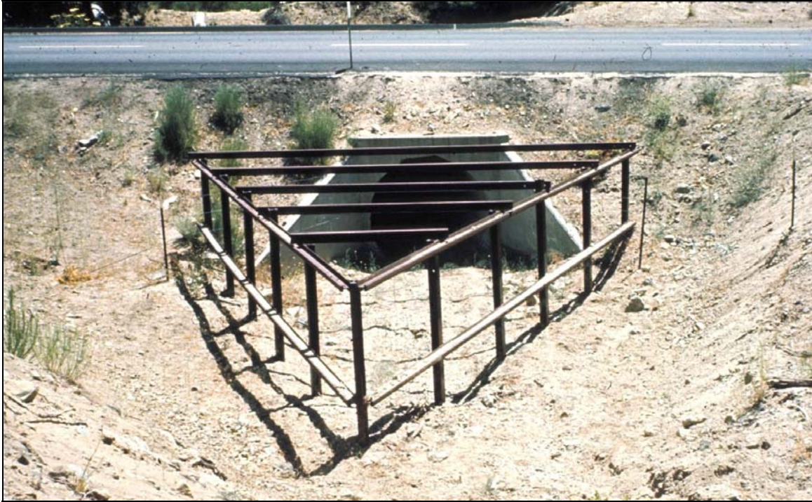
Figure 5.2. Steel rail debris deflector (looking downstream).
