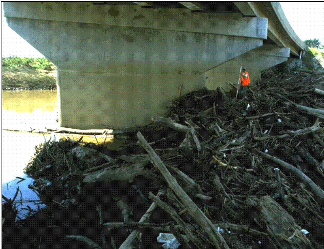
Figure 2.6. Debris accumulation at a bridge structure. (17)
