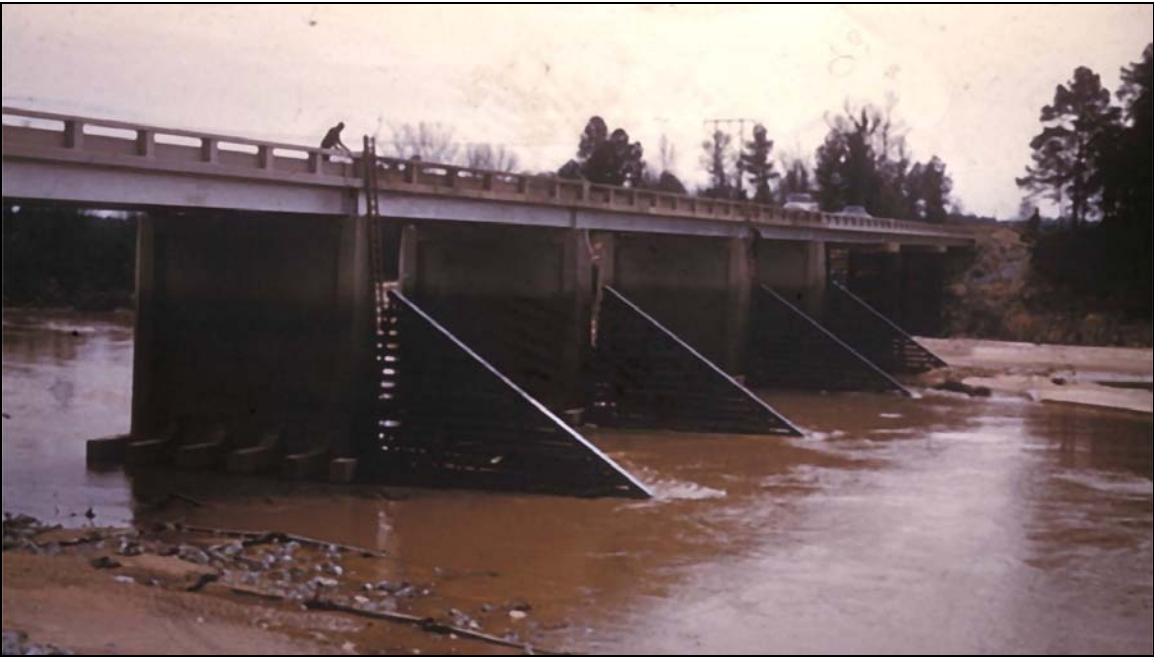
Figure 5.35. Timber debris fins with sloping leading edge.
