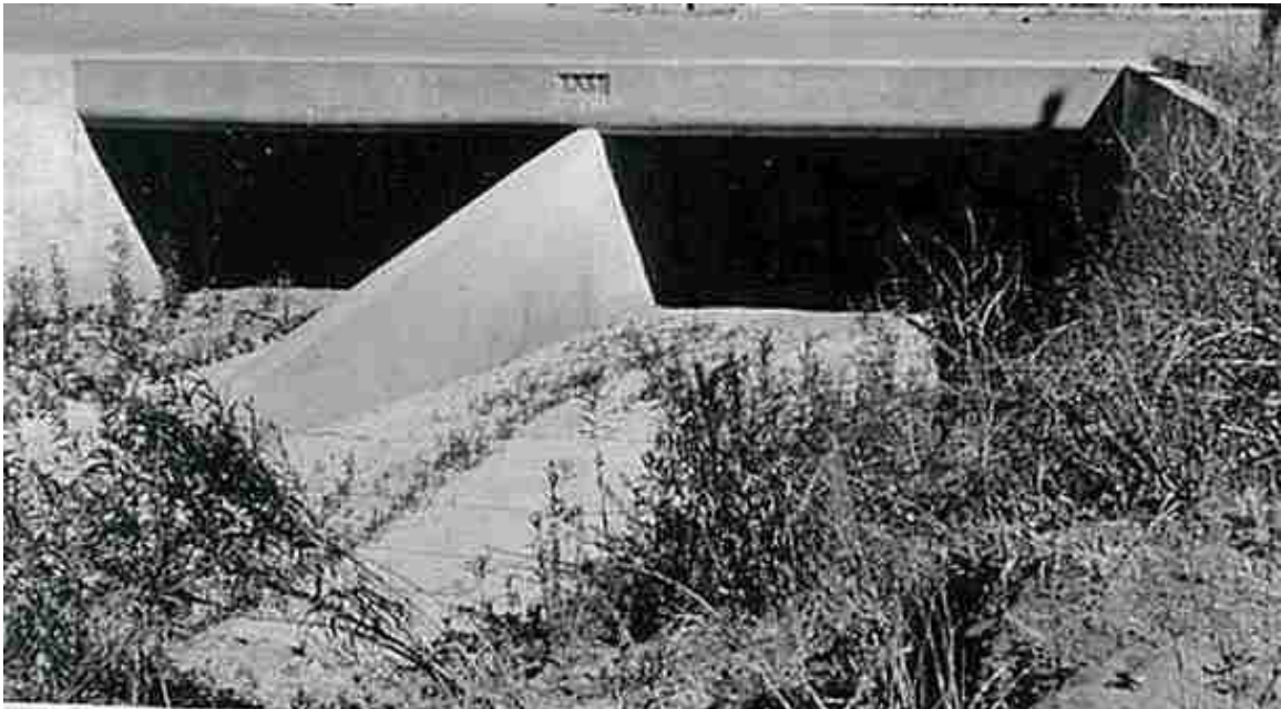
Figure 5.30. Concrete debris fin with sloping leading edge as extension of center wall.
