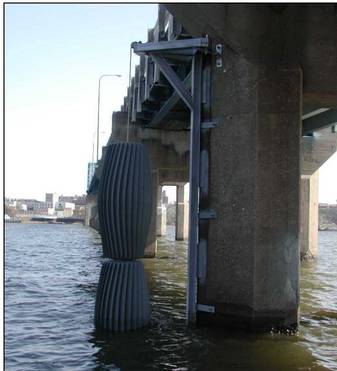
Figure 5.47. Close up of double-stacked installation debris sweeper on Interstate 24 over the Mississippi River.
