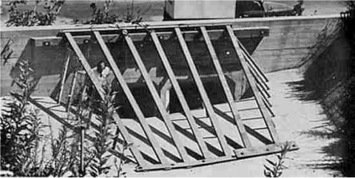
Figure 5.21. Steel grill debris rack with provision for cleanout afforded by concrete paved area in foreground.
