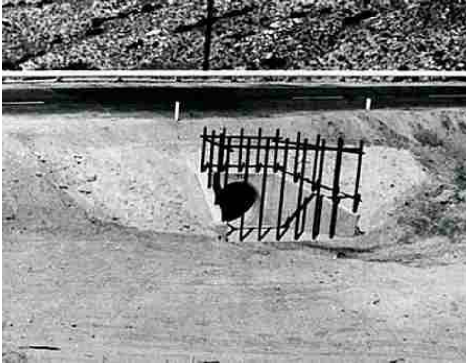
Figure 5.17. Rail debris rack in arid region (see Figure 5.18).
