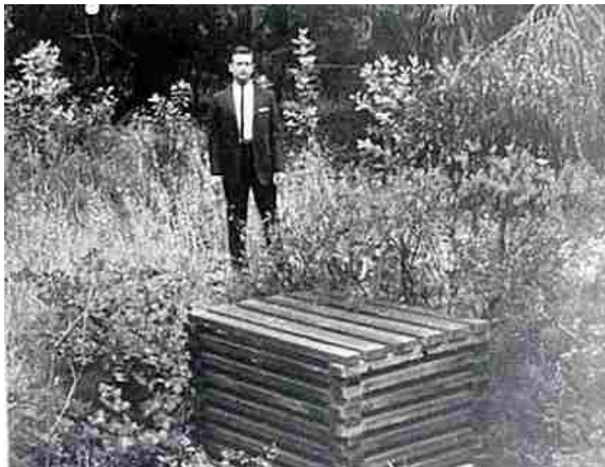
Figure 5.28. Redwood debris crib with spacing to prevent passage of fine material. Basin had buildup of 30 feet.
