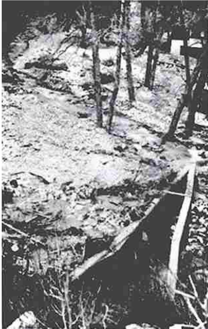
Figure 5.9. Timber pile debris deflector protected culvert during heavy floods. Nearby culverts without deflectors were plugged.
