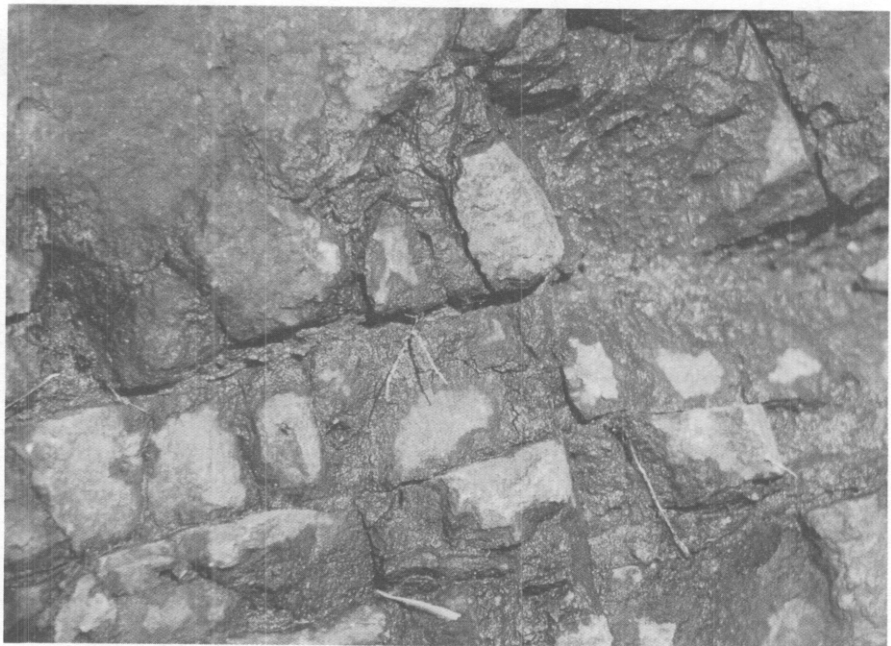
Figure 5.21 Weathered joint surface. Note the red colored clay between the rock surfaces.
