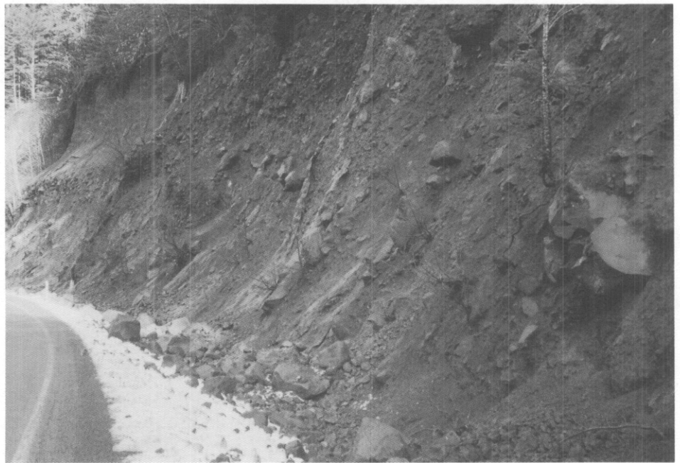
Figure 5.25 Oversteepened soil/rock slope
