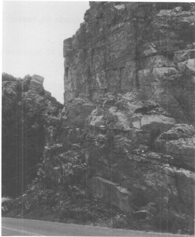
Figure 5.5 The launch feature midway up the slope adds to the ineffectiveness of this narrow roadside ditch.
