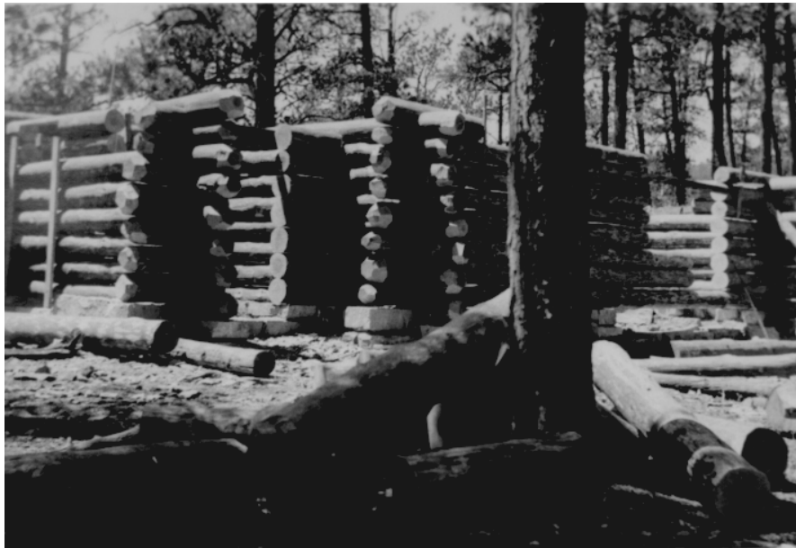
Figure 2. "Ranger Cabin Under Construction, 1935." View to the northwest showing near-completion of wall logs. Jewel Cave NM photo archives, Neg. No. 2793.
