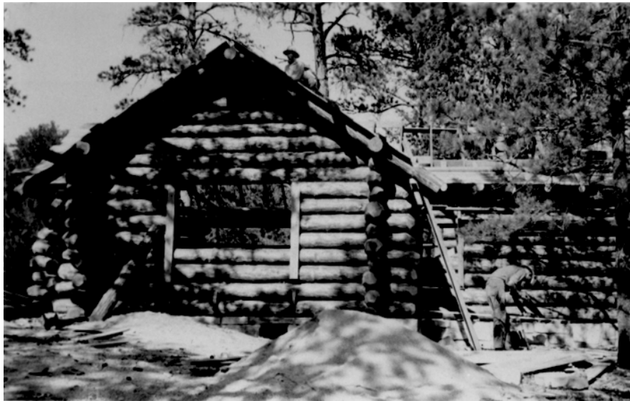
Figure 3. The Ranger Station during construction, 1935, view to the east. Note that the gable end logs and roof framing have been completed. Jewel Cave NM photo archives, Neg. No. 844.
