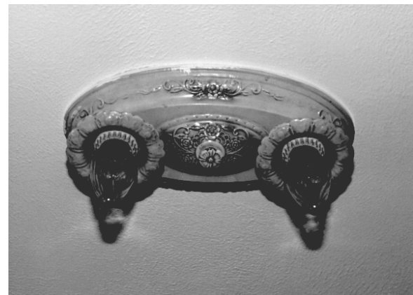
Figure 27. Ceiling fixture at CCC structure, Wind Cave National Park. A similar fixture may have been in the Ranger Cabin. Photo by Laura Johnson, 1997.
