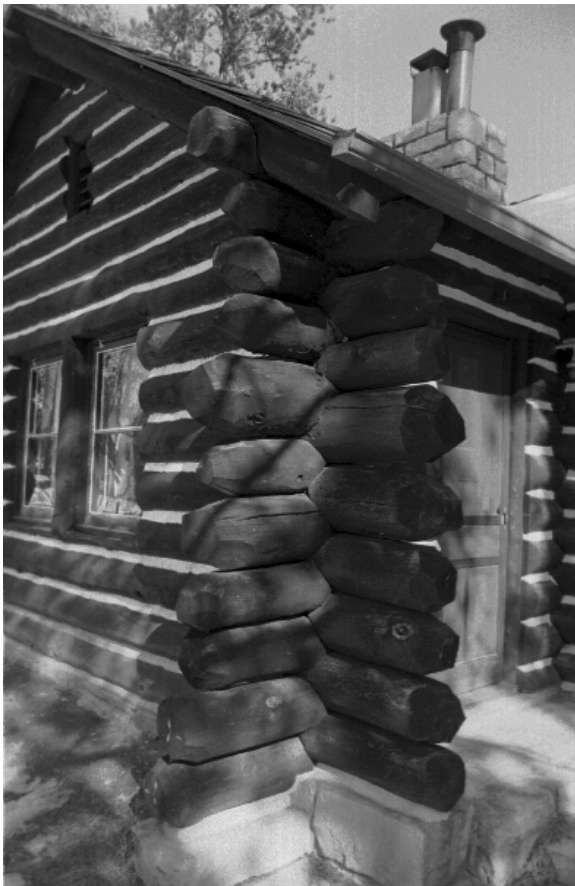
Figure 23. Log crowns at southwest corner of kitchen wing. Photo by the author.
