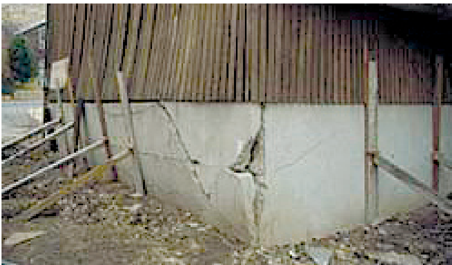
Figure 38. Cracking of the foundation of a structure. (Photograph courtesy of Utah Geological Survey.)
