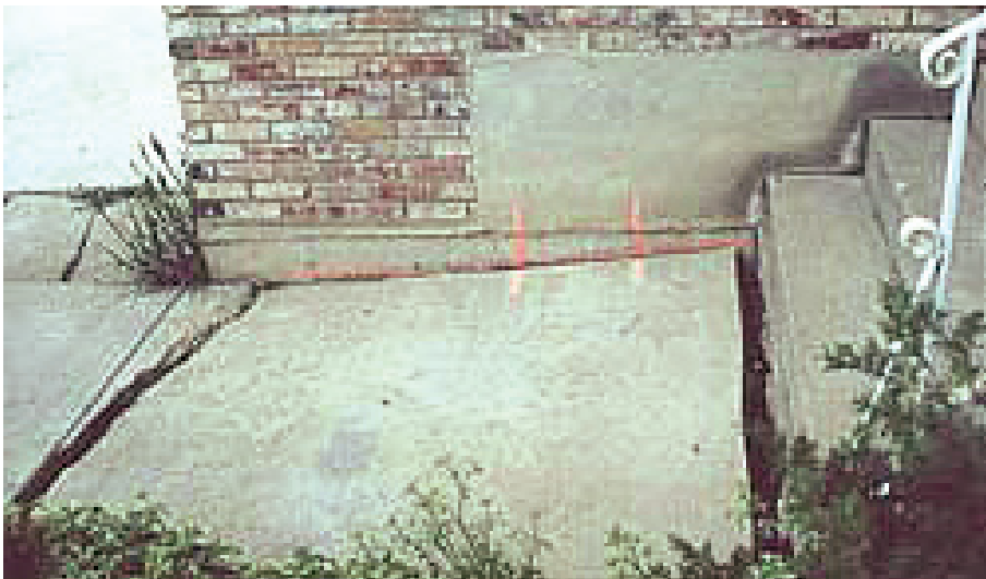
Figure 37. Sidewalk pulling away from house. (Photograph courtesy of Utah Geological Survey.)
