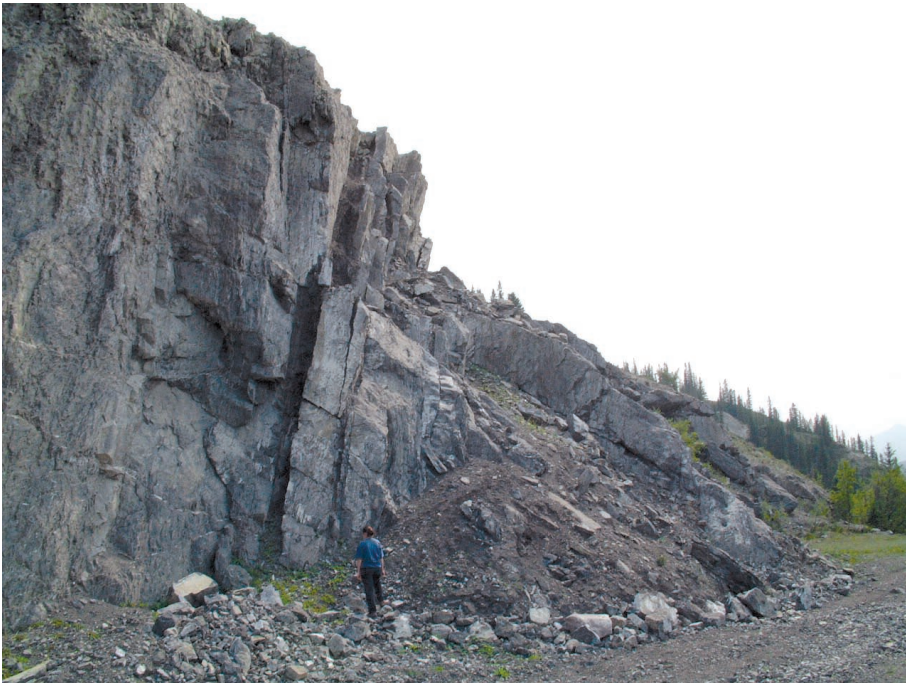
Figure 6. Photograph of block toppling at Fort St. John, British Columbia, Canada. (Photograph by G. Bianchi Fasani.)
