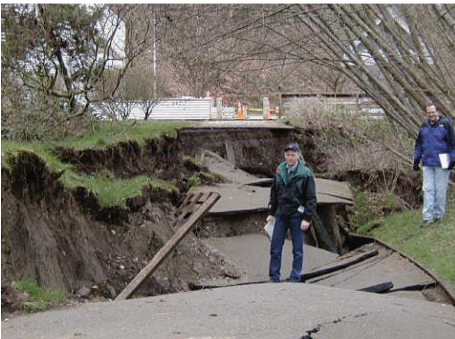
Figure 25. Lateral spreading damage. Photograph shows the Puget Sound area in Washington, USA, after the 2001 Nisqually earthquake. (Photograph courtesy of the Seattle Times.)
