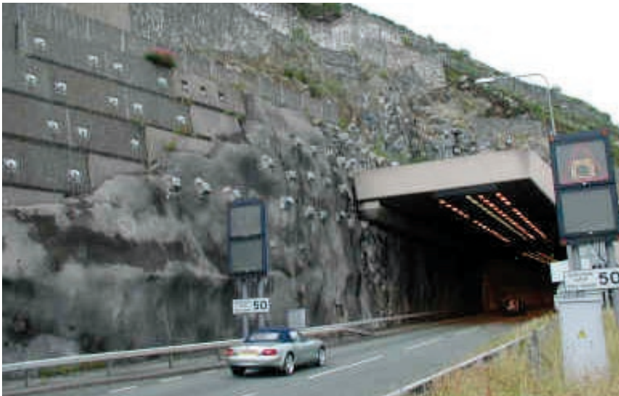
Figure C20. This photograph shows rockfall countermeasures that include mass concrete retaining walls, gabion walls (both wall types are at top of photograph), check fences, boulder treatment, and buttressing. (Photograph is the Pen-y-Clip tunnel on a highway in North Wales, United Kingdom. Photograph by Dave Giles, Engineering Geology Consultancy Group, University of Portsmouth, United Kingdom.)
