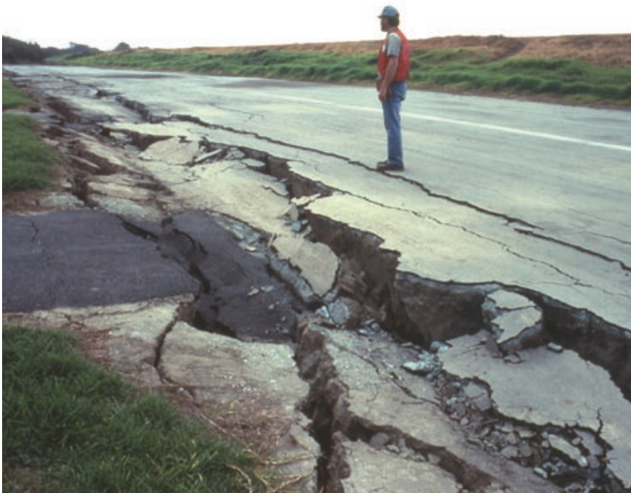
Figure 12. Photograph of lateral spread damage to a roadway as a result of the 1989 Loma Prieta, California, USA, earthquake. (Photograph by Steve Ellen, U.S. Geological Survey.)
