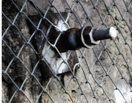
Figure C32. Closeup photograph of a rock anchor on a rock face, with mesh over the surface for more protection. The anchor is set in the rock about 5 meters (15 feet) deep.
