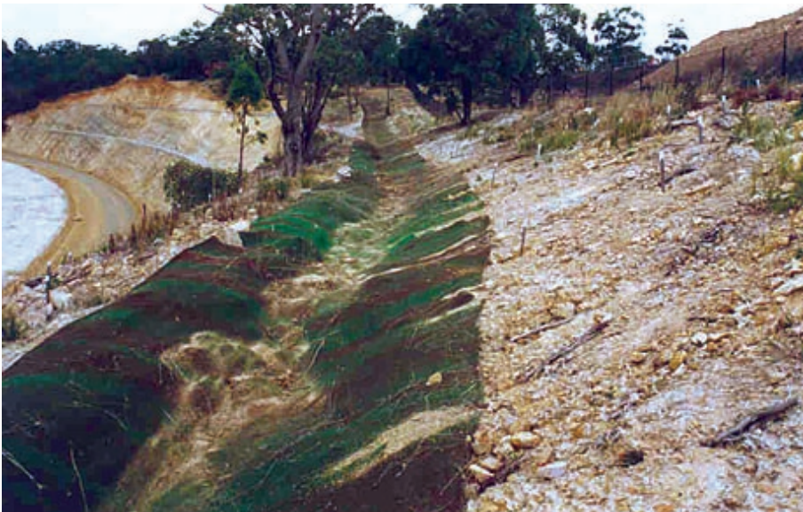
Figure C9. Schematic and photograph of a drain trench. (Graphic from Reference 11, photograph by Department of Transport, Energy and Infrastructure, South Australia.)
