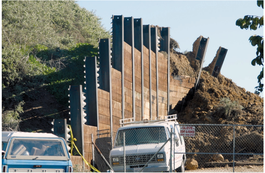
Figure C36. Caution is required in locating and constructing debris-flow retaining walls. This photograph shows a steel-and-timber retaining wall built at La Conchita, California. This wall was built to protect houses after a 1995 landslide but was partially destroyed by a debris flow that occurred in 2005 in the same area. The wall protected some structures, but it was severely damaged, and the partially deflected material damaged another house. (Photograph by Randall Jibson, U.S. Geological Survey.)
