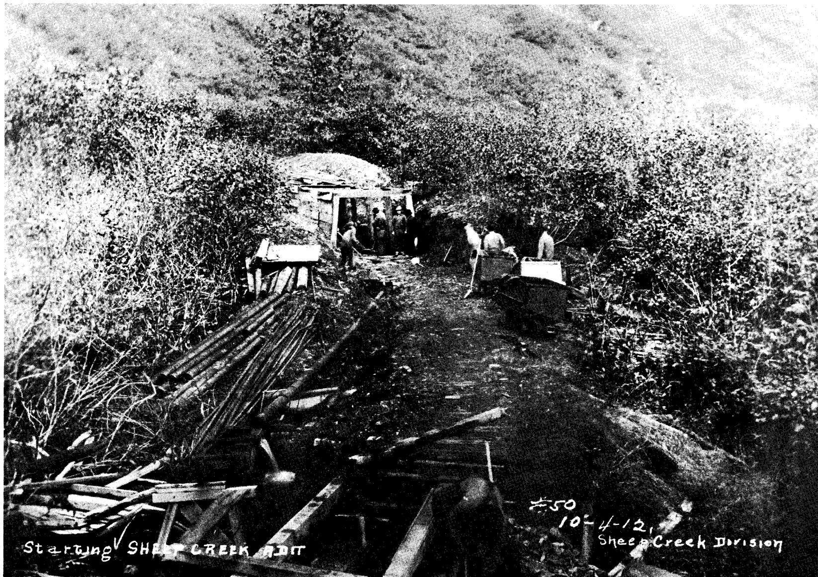
Figure 18. Beginning the 10,400 ft-long Sheep Creek Tunnel in 1912 which would connect with the Perseverance mine (Winter & Pond Coll., Alaska Historical Lib.)
