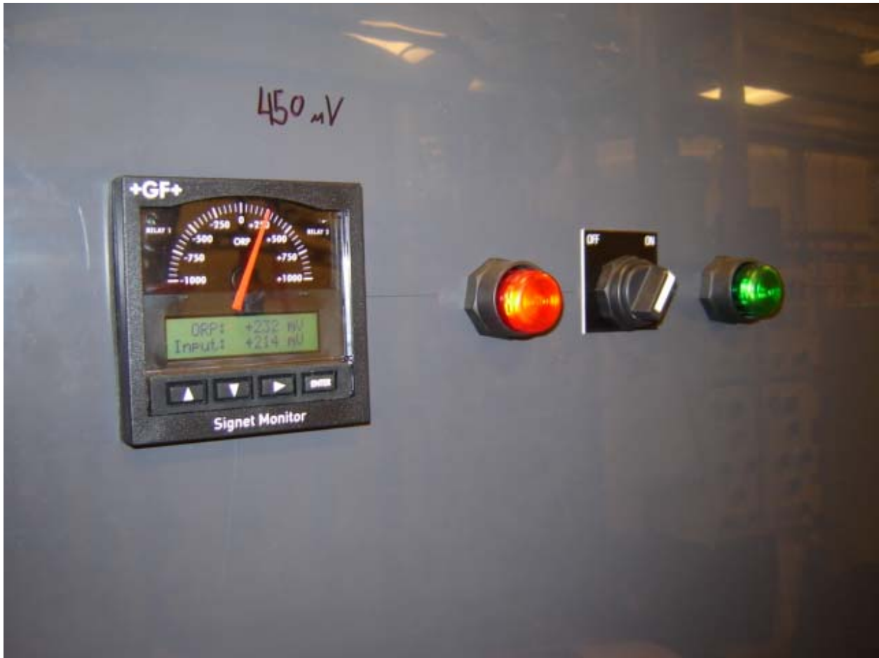
Figure 2-3. ASOP ORP meter display and system power switch on cabinet door.
