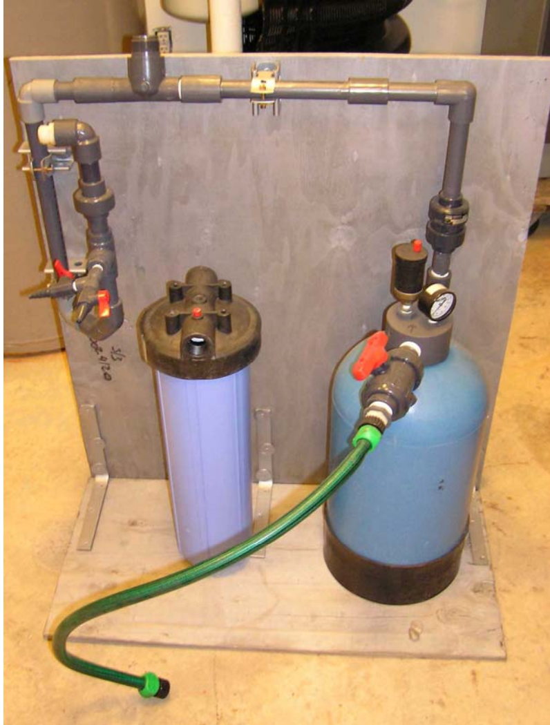
Figure 2-2. ASOP module ozone contact tank and activated carbon filter.
