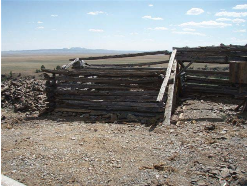
Lander Field Office – Carrie Shields Mine project; this is the shaft area that was capped and grated to allow bats in and out. The cable would have come up from the shaft and been attached to the top of the whim shown in the next picture.
