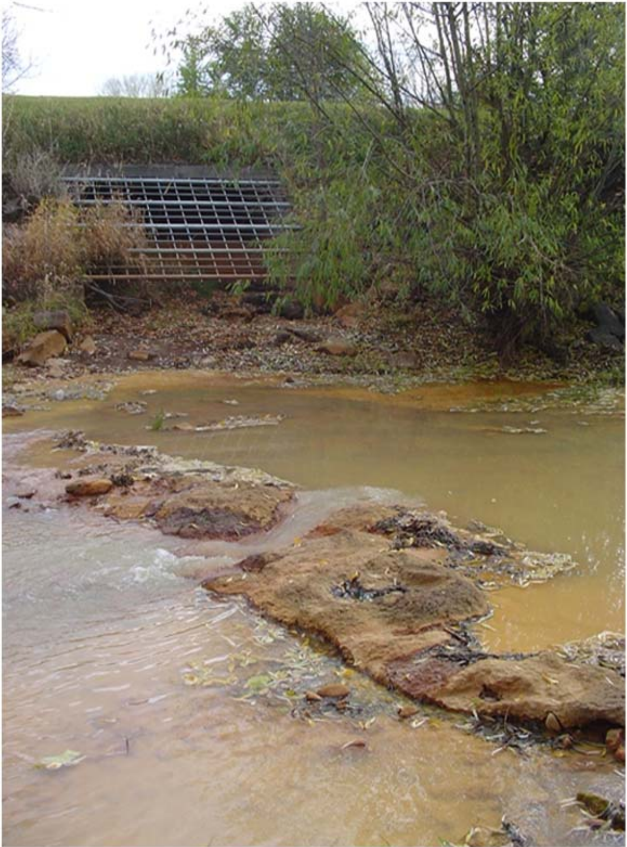
Figure 15. Outlet of the Lewis Coulee Storm Drain where it enters Belt Creek.
