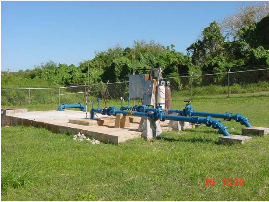
Figure 1. Saipan's pumping station, Kagman area.
