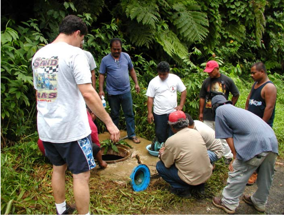
Figure 1 Students performing field maintenance on pressure regulating valve
