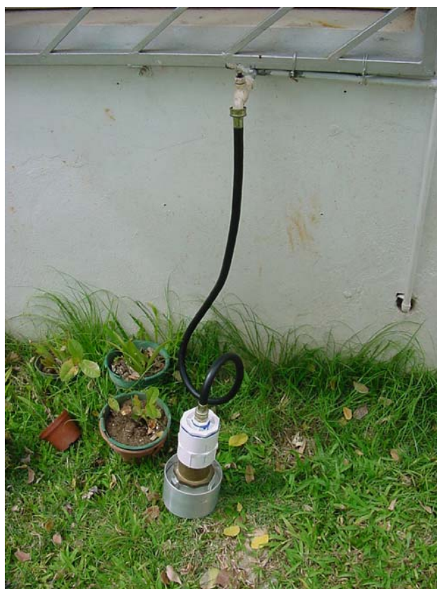
Figure 5.4. Pressure meter at the household entrance
