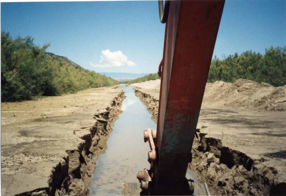
Figure 3. Pilot channel being excavated through a previously formed sediment plug (August 1991 photo).
