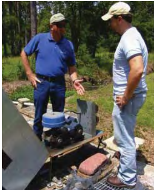
Lake Pontchartrain Basin Foundation has worked to train sewer operators to reduce discharges from lagoons and small package plants.
