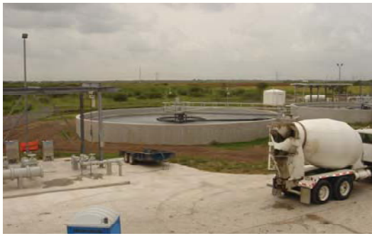
San Benito Wastewater Treatment Plant Photos: José Rodríguez, EPA Region 6
