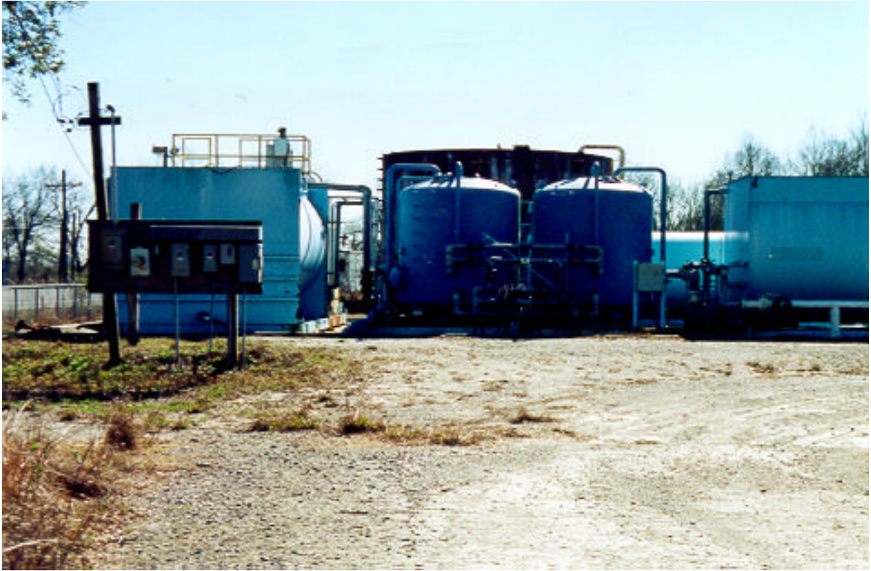
Carbon adsorption water treatment unit constructed during the Remedial Action, Phase I. (1990 -1992)
