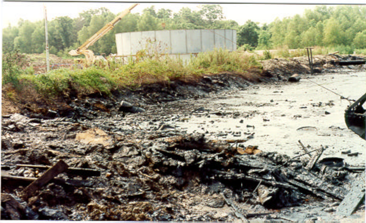
Both photos show on-site lagoon #1 during the Remedial Action, Phase I. Removal of existing lagoons, abandoned tanks and structures, construction of a lined impoundment, land treatment or bioremediation unit and a carbon adsorption water treatment unit. (1990 - 1992)
